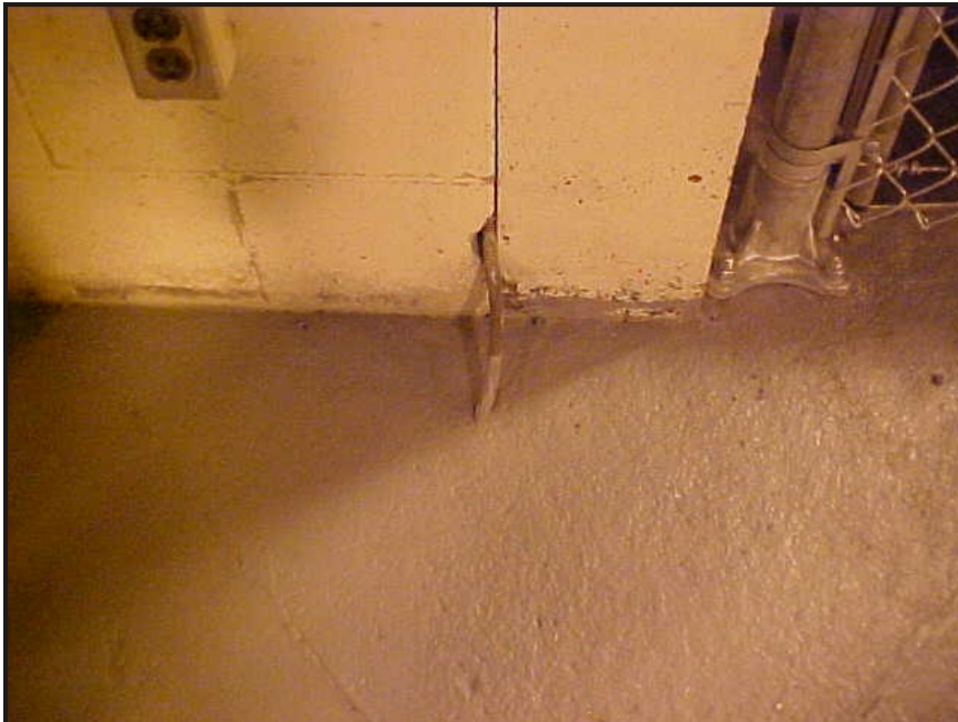
(24) Photo of a building grounding cable in the maintenance shop area
