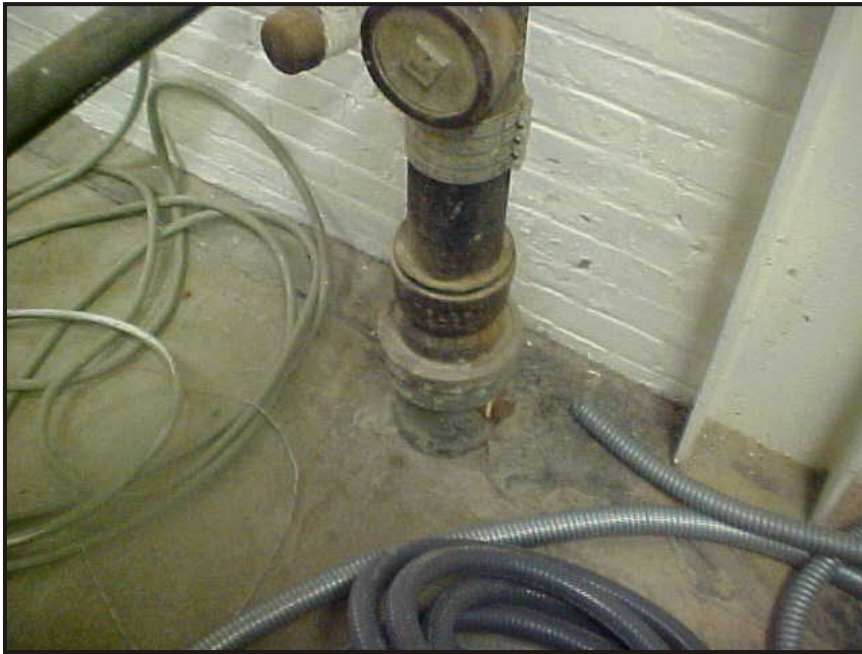
(3) Photo of a roof drain in the server room
