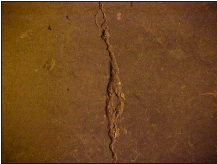
(13) Photo of a superficial crack in the floor in the mechanical room at the south end of the building
