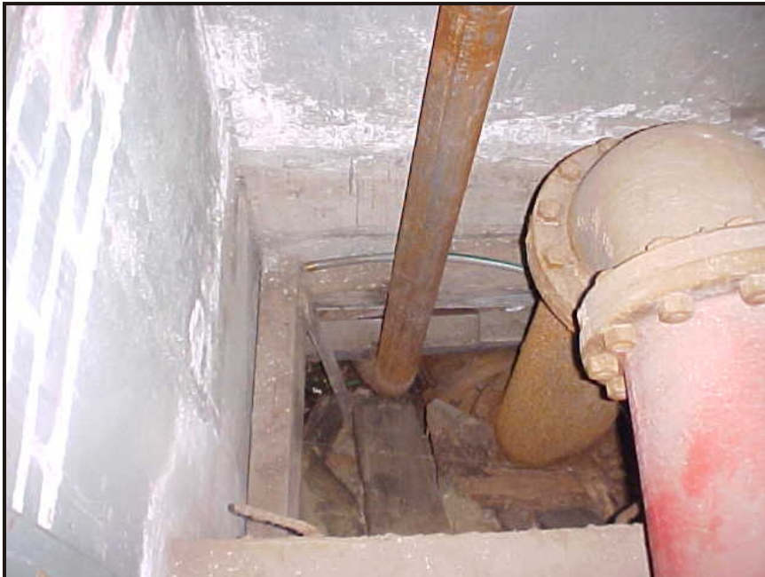
(24) Photo of a fire pump pit located just off the compressor room at the northeast corner of the building
