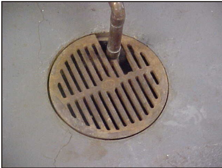
(7) Photo of a floor drain in the South Central section of the mechanical room
