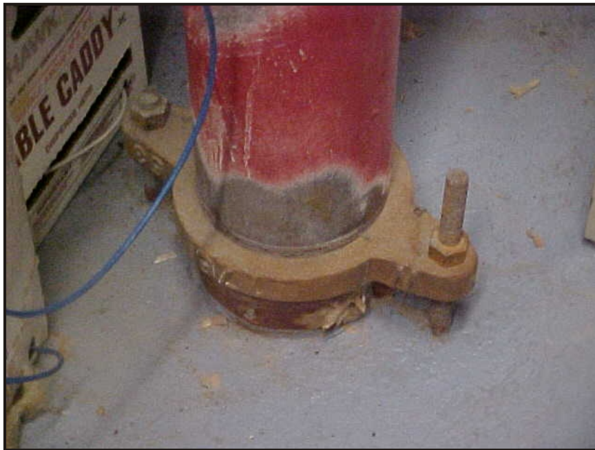
(13) Photo of a fire riser in the health and safety records storage room
