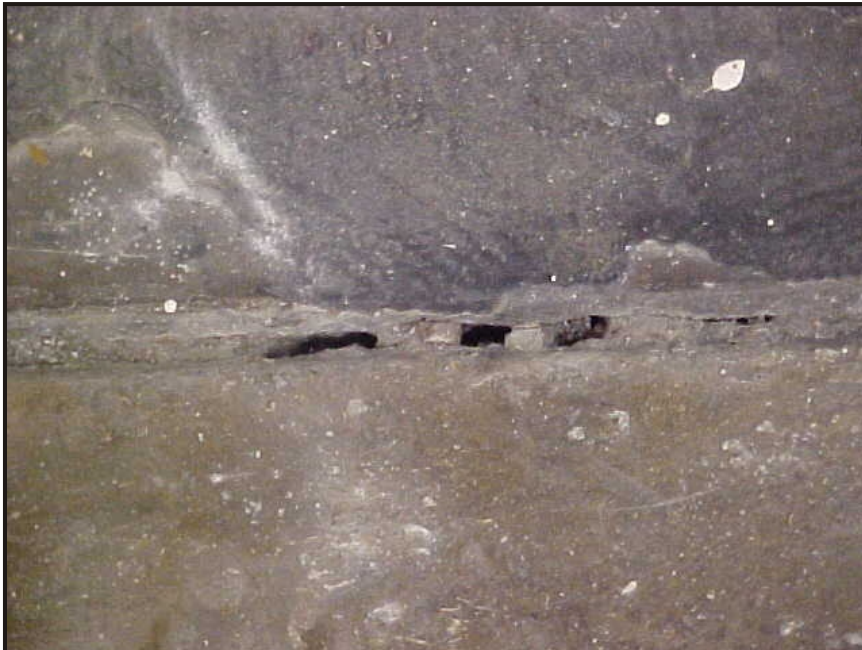
(4) Photo of a crack in the concrete floor on the north wall of the server room that appears to be superficial with an apparent depth of 2-3"
