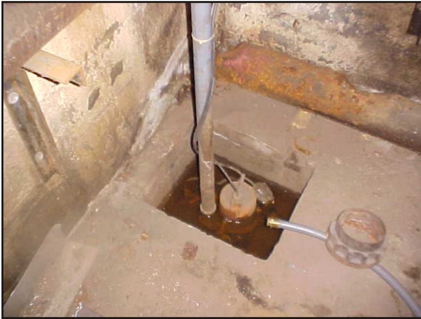
(23) Photo of a sump pump pit located in the lower level of the compressor room at the northeast corner of the building
