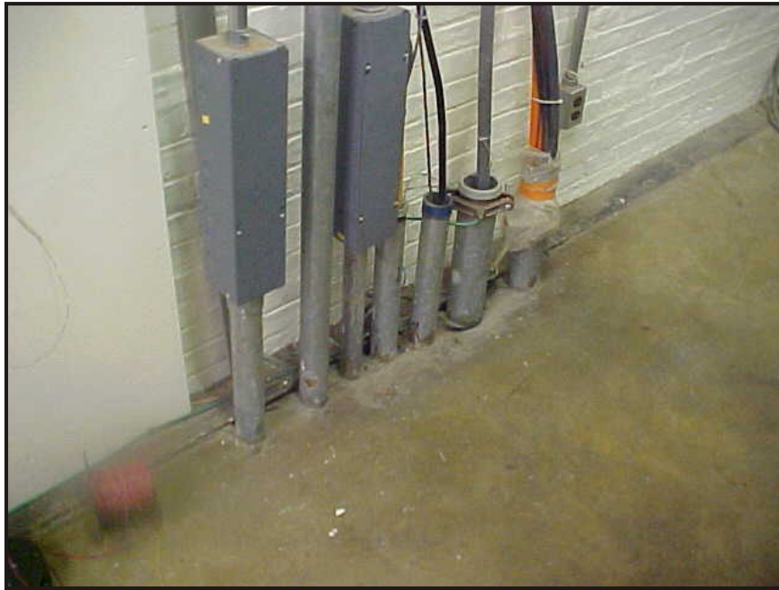
(1) Photo of several conduits in the server room
