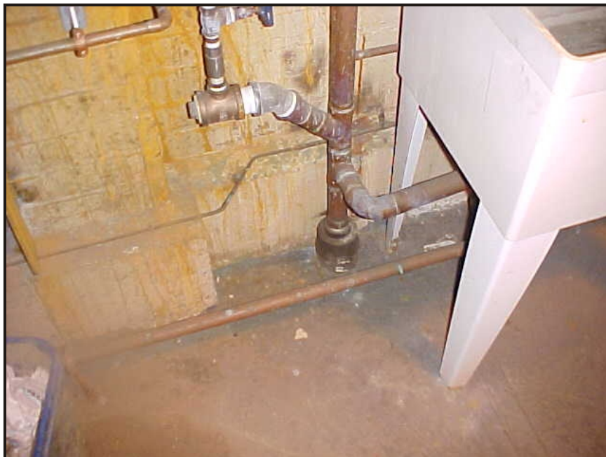
(12) Photo of a sink drain line in the mechanical room at the south end of the building
