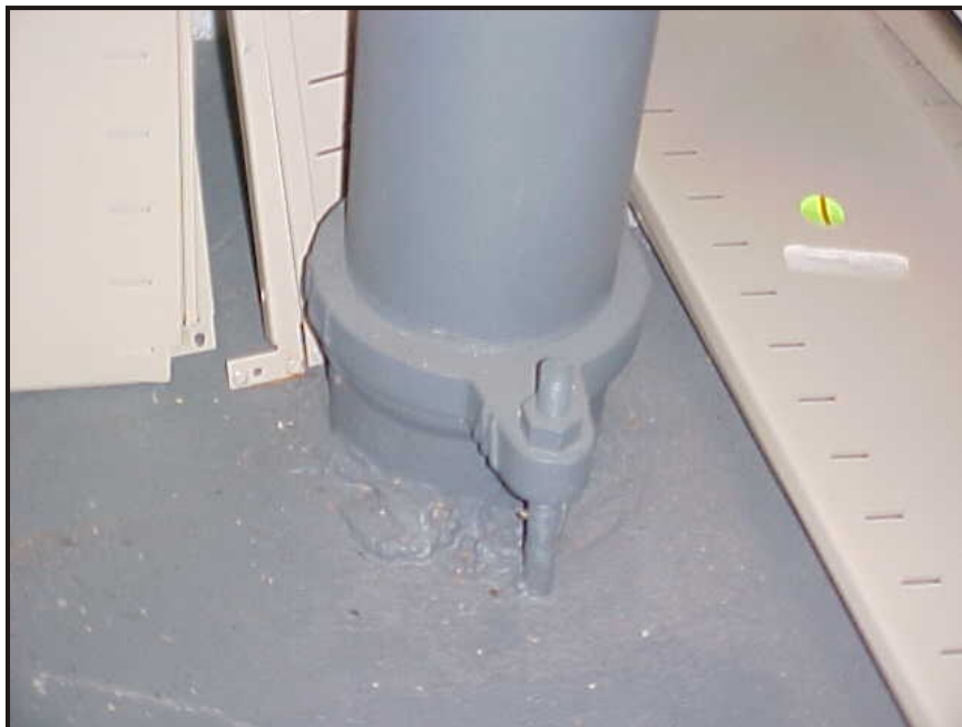
(12) Photo of a fire riser in the insurance claims storage room
