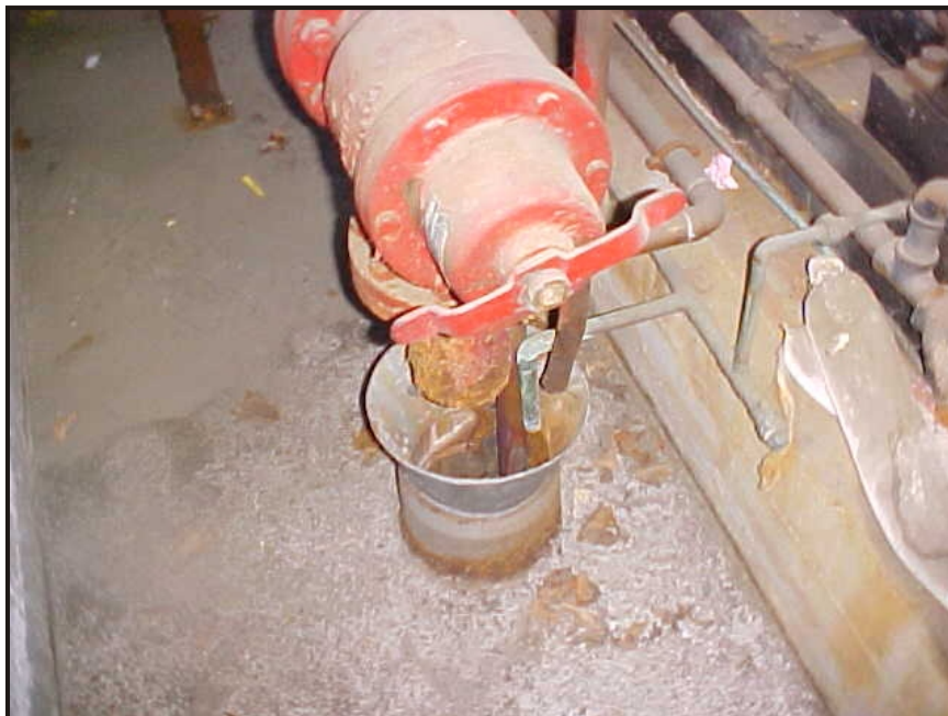
(25) Photo of a fire line drain in the fire pump room just off of the compressor room at the northeast corner of the building
