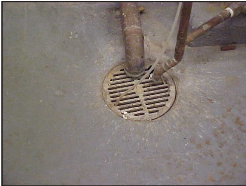
(11) Photo of a floor drain in the southwest section of the mechanical room
