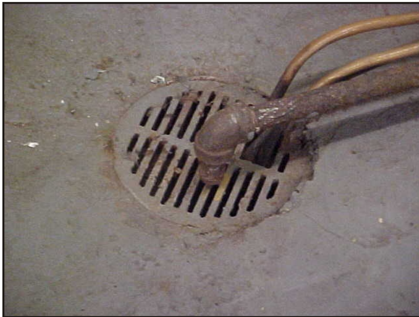
(5) Photo of a floor drain in the northeast section of the mechanical room
