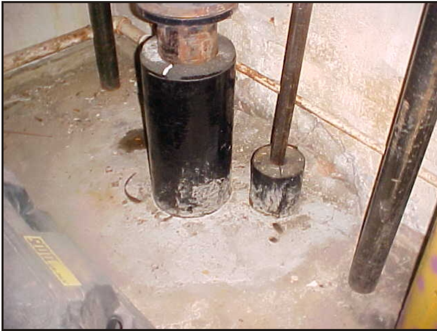
(7) Photo of a steam line in fire equipment storage area
