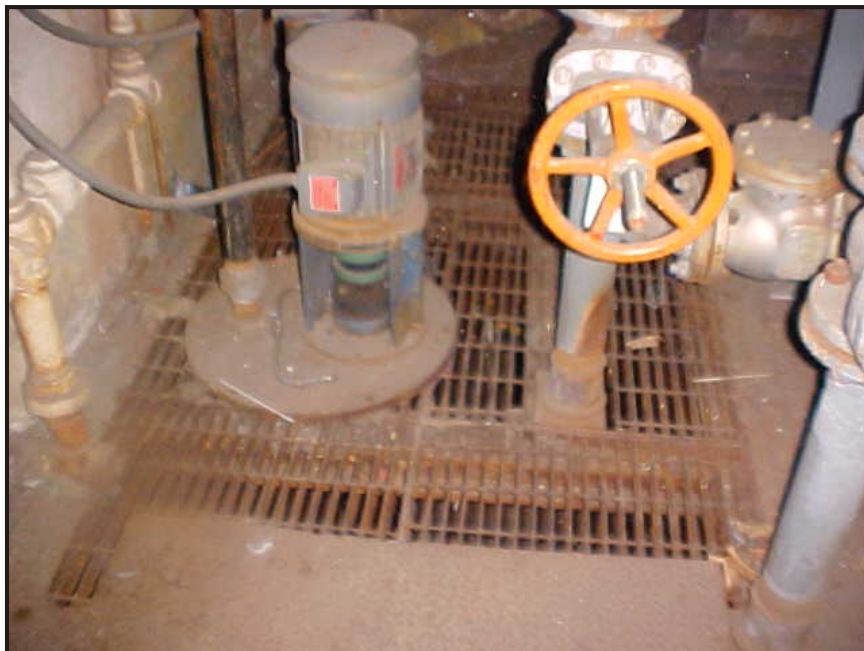
(20) Photo of a pump pit located below a steel grated area in the old boiler room at the northeast end of the building
