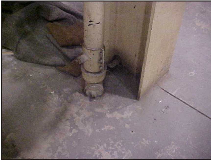
(17) Photo of a roof drain in the high bay storage area at the northwest corner of the building
