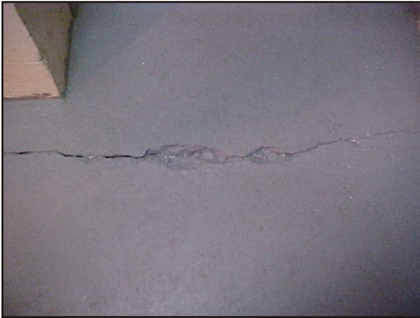
(19) Photo of a superficial floor crack in front of the southeast exit door of the records storage area.
