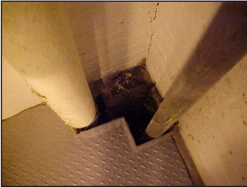
(25) Photo of two (2) steam pipes that go through a steel grated plate in the northeast corner of the maintenance shop area*
