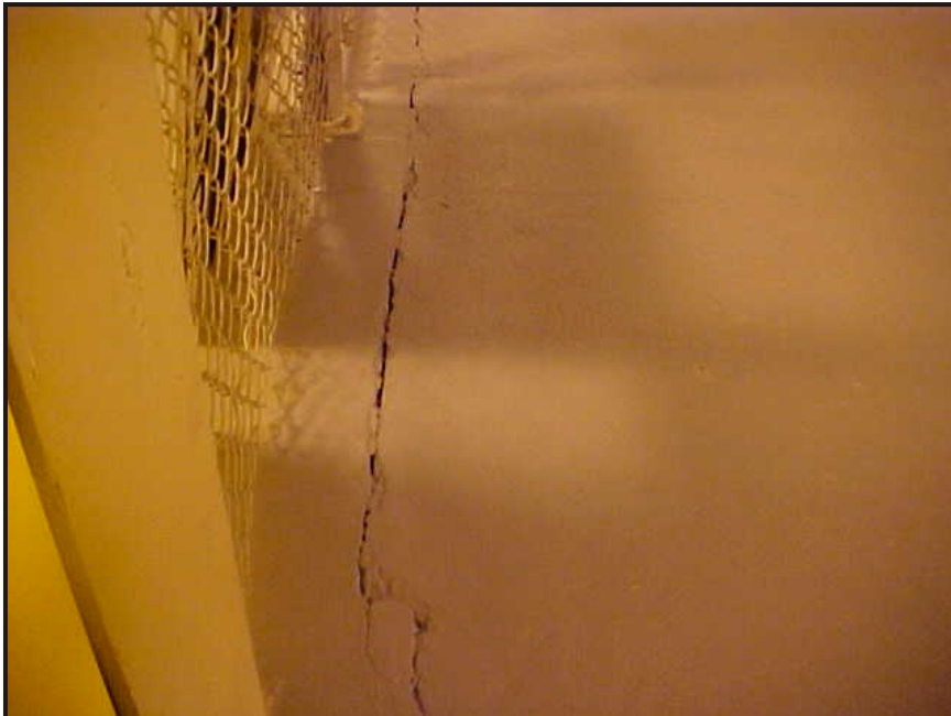
(20) Photo of a superficial crack in the concrete floor that runs from north to south in front of the mechanics crib
