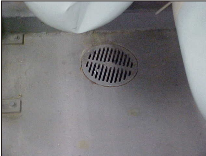
(10) Photo of a floor drain in the center of the mechanical room
