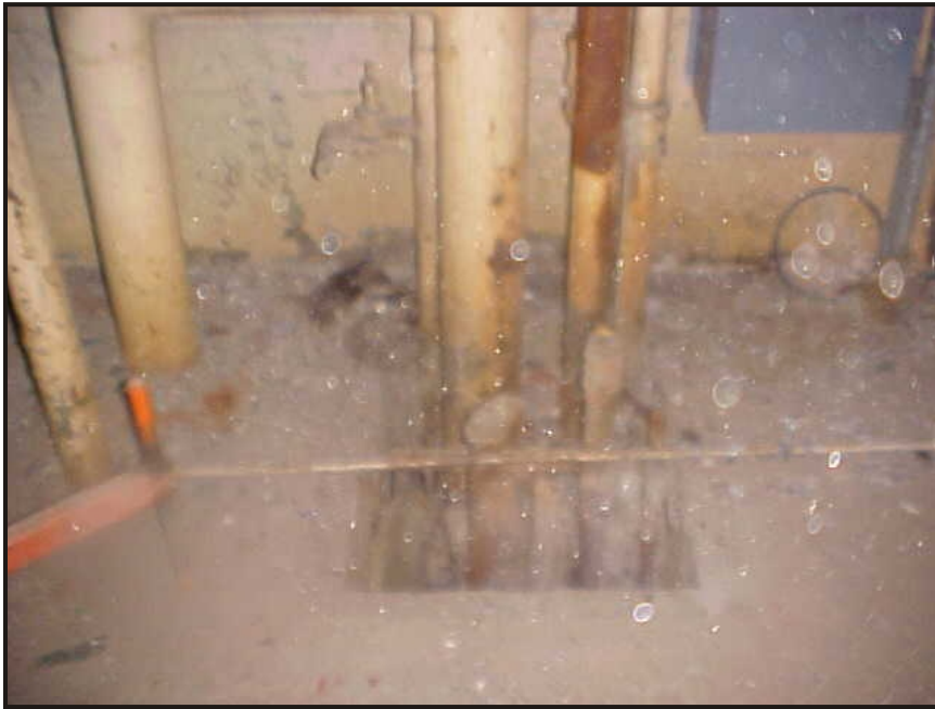
(21) Photo of an open pipe chase in the old boiler room at the northeast end of the building
