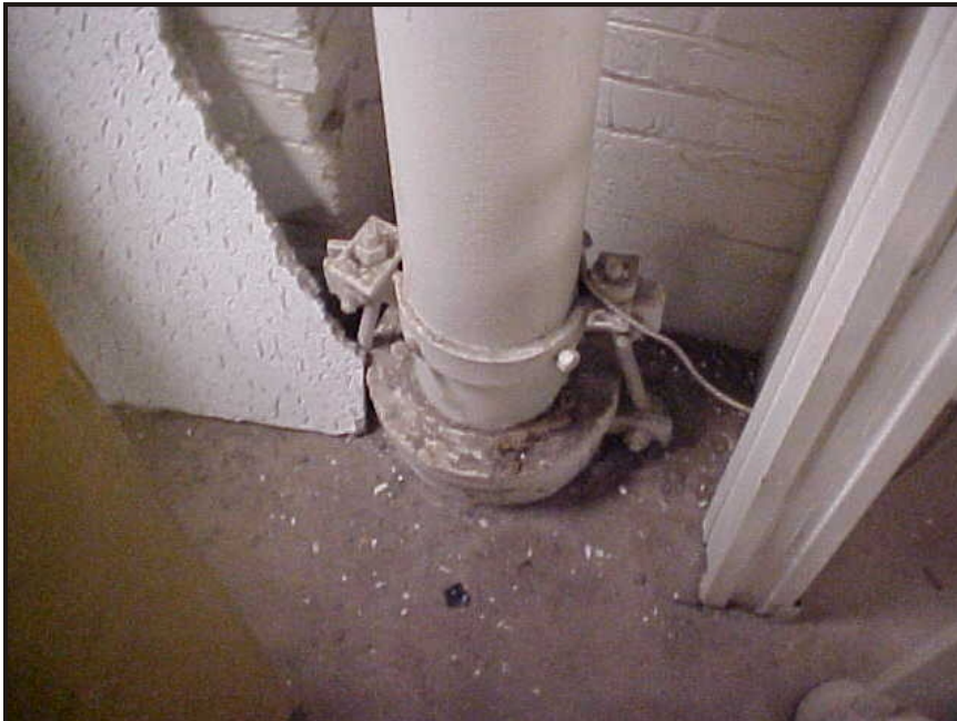
(8) Photo of a fire riser (51-8B) in empty storage area
