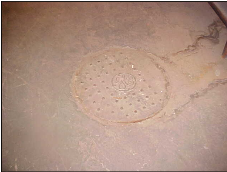
(9) Photo of a sewer manhole cover in the mechanical room at the south end of the building
