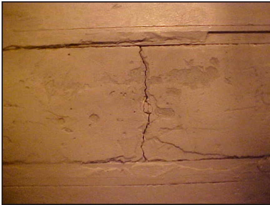
(17) Photo of a superficial floor crack on the east end of the fenced in records storage area in front of the double fenced gate
