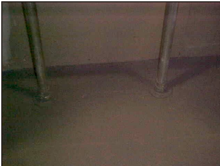
(14) Photo of electrical conduit in the MCC room
