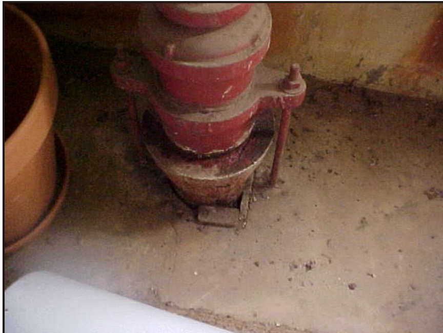
(14) Photo of a fire riser in the high bay storage area at the northwest corner of the building
