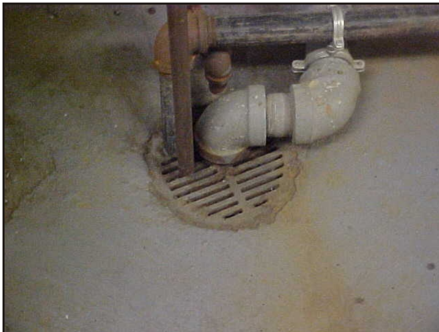
(8) Photo of a floor drain in the North Central section of the mechanical room
