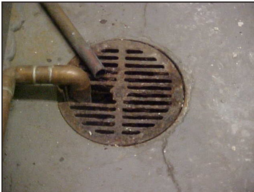
(6) Photo of a floor drain in the southeast section of the mechanical room
