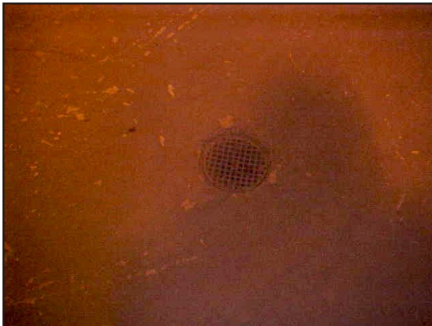
(10) Photo of a floor drain in the mechanical room at the south end of the building, several others floor drains were also present in this room
