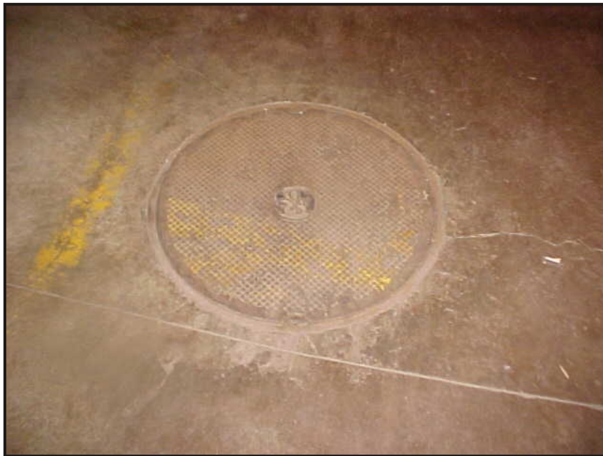
(5) Photo of an electrical manhole cover just north of the new boiler
