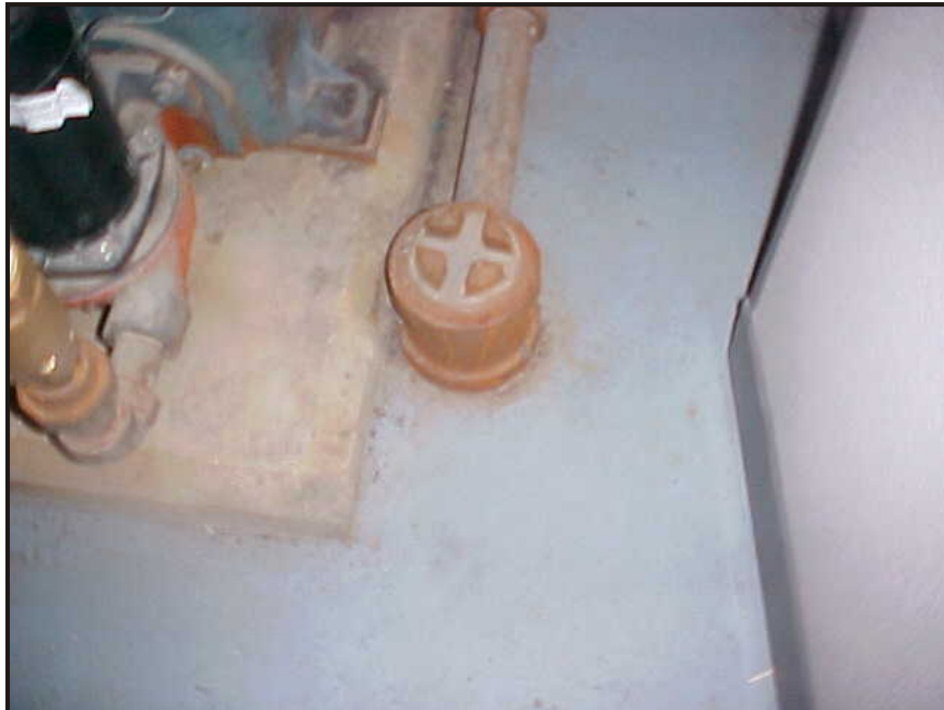
(18) Photo of a condensate pump drain in the electrician's storage area
