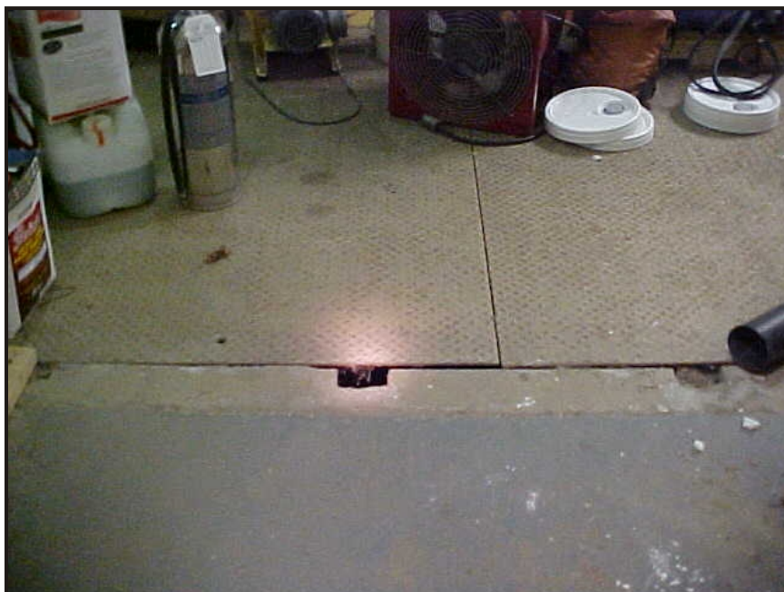
(6) Photo of a representative steel plated area covering a 4-foot vault, several other vaults were also present in this room
