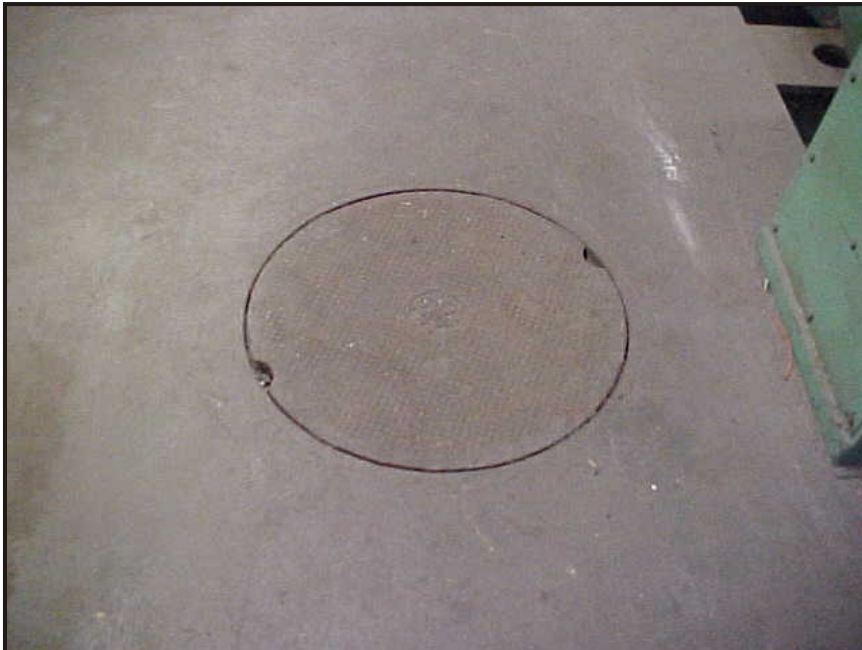
(22) Photo of generator access manhole cover in the compressor room located at the northeast corner of the building
