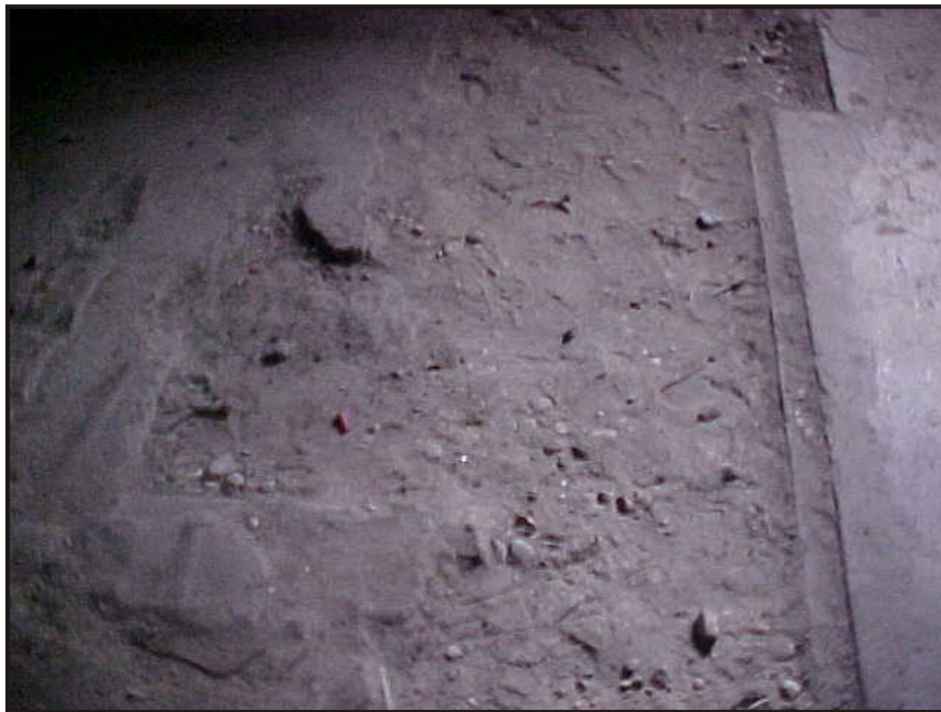
(19) Photo of representative open gravel floor area in the old boiler room at the northeast end of the building
