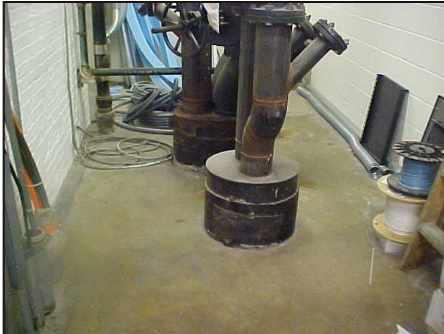
(2) Photo of the chiller water piping in the server room
