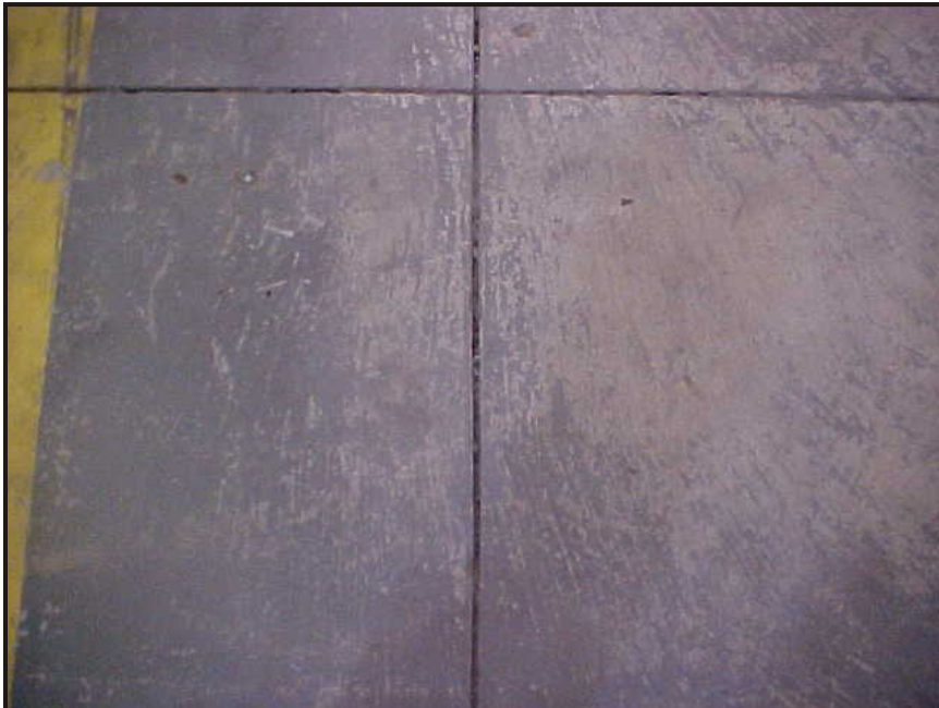
(18) Photo of expansion cracks in the floor located in the high bay storage area at the northwest corner of the building
