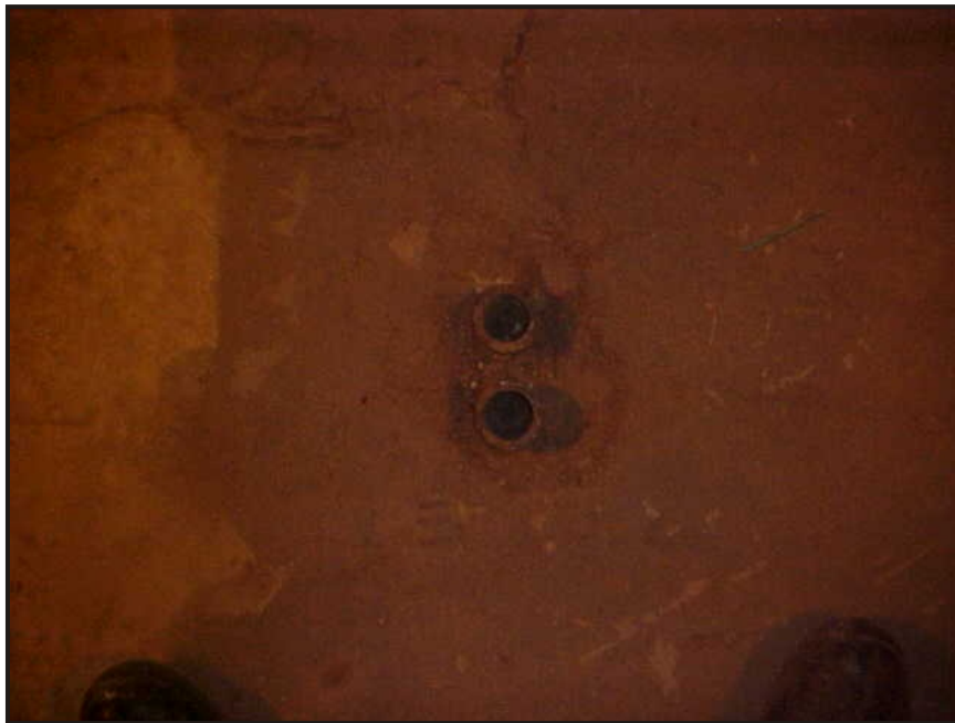
(11) Photo of sealed conduit holes in the mechanical room at the south end of the building
