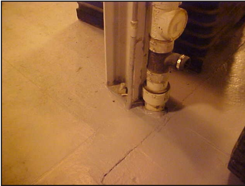
(23) Photo of a roof drain on the side of a steel beam in the maintenance shop area
