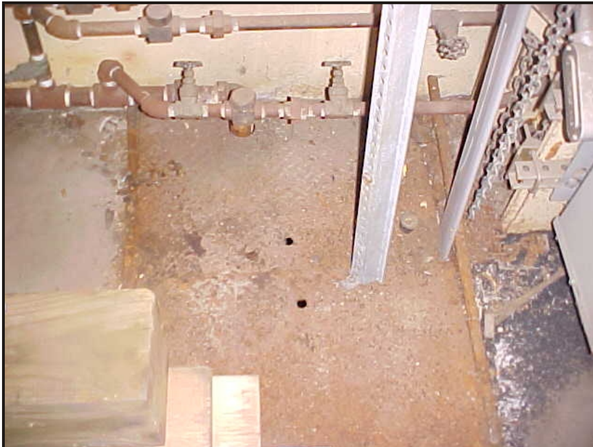
(16) Photo of a steam line pit under steel grating in the high bay storage area at the northwest corner of the building
