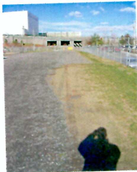
Photo #8: Absence of Vegetative Cover East of Gravel Parking Area (11/18/05)
