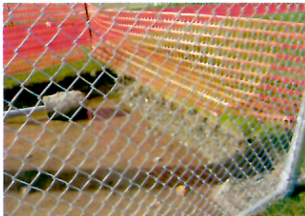
Photo #3: 1st Base Dugout. Excavation in Advance of Dugout Construction. Note approximate excavation depth (12 inches) and standing water (11/18/05)
