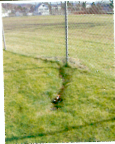
Photo #6: Erosion Gully with Soil Cover Area Along Southern Fenceline of Ballfield Area Note Soil Deposit on Far Side of Fenceline (11/18/05)
