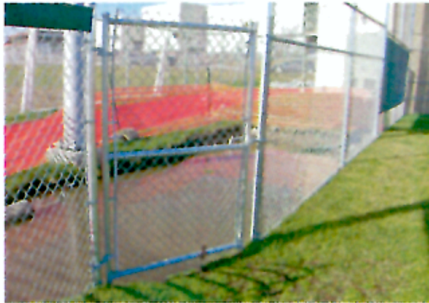
Photo #2: 1st Base Dugout. Excavation in Advance of Dugout Construction. Note approximate excavation depth (12 inches) and standing water (11/18/05)
