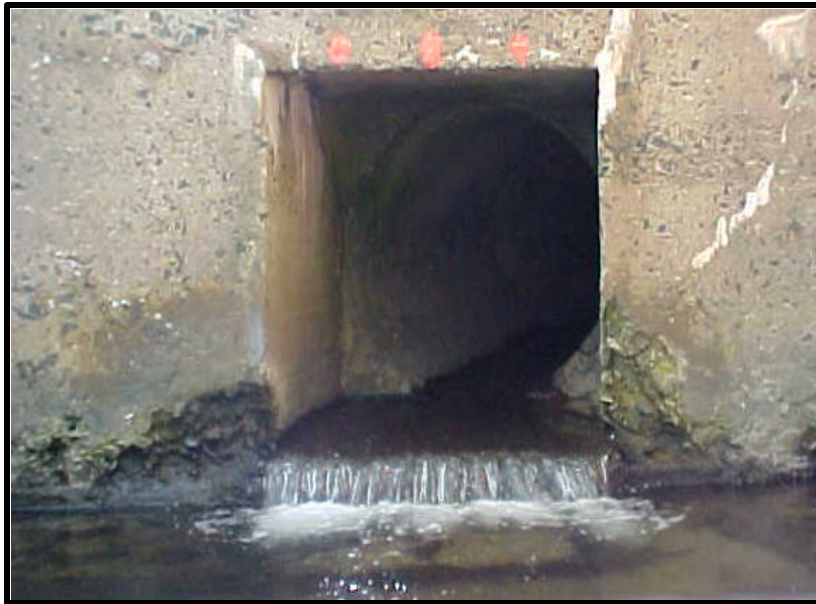
Outfall A: Looking upstream into culvert. Orange stripes designate locations for velocity measurements
