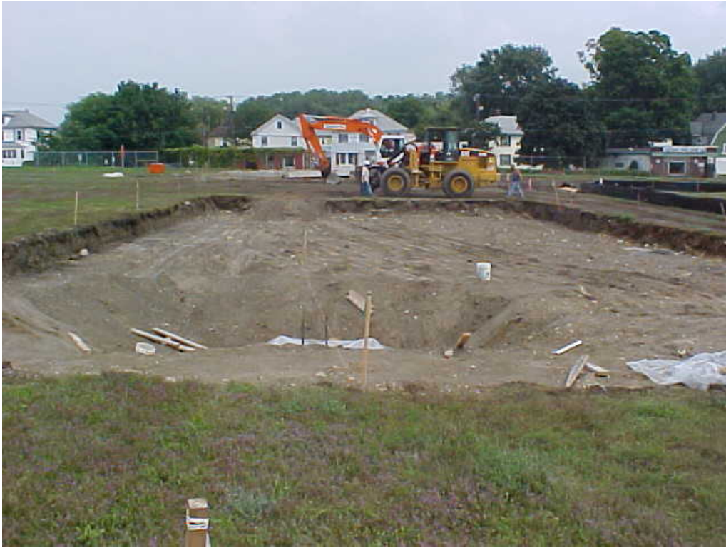
Photograph 11 Area of 2-foot removal along the southern edge of the CRA following excavation. Photo taken looking east.
