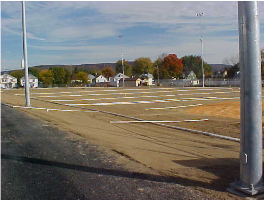
Photograph 18 Installation of the irrigation system in the field area. Photo taken looking southeast.
