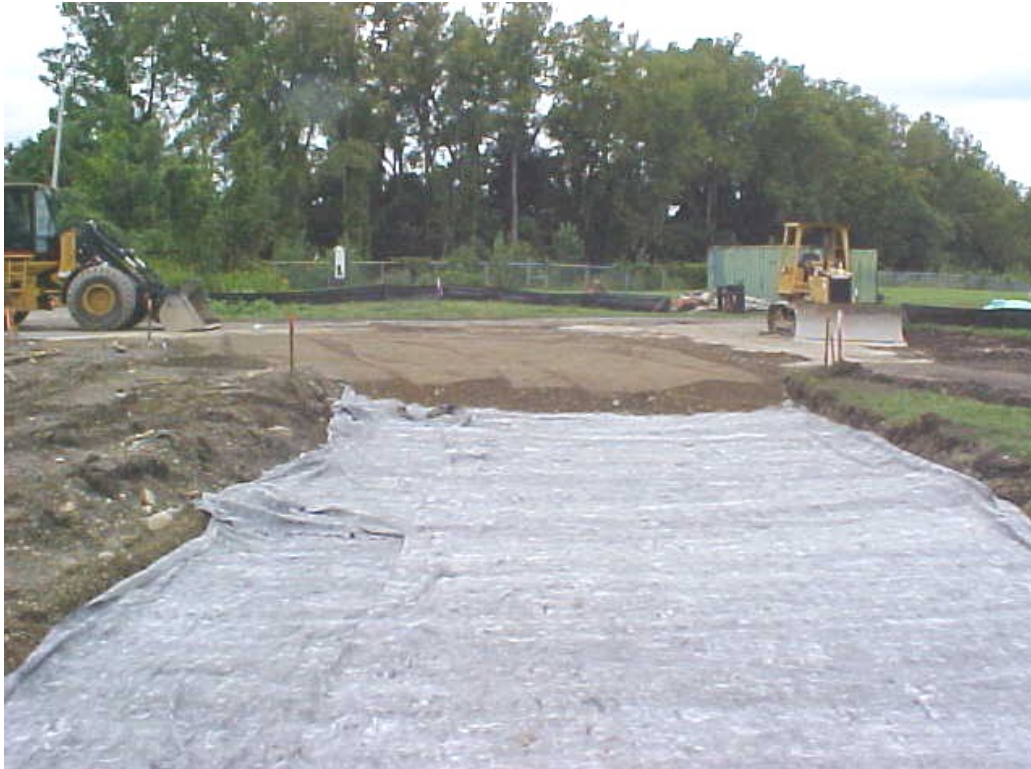
Photograph 15 Woven geotextile placed on the subgrade of the new access road. Note the placement of gravel over the geotextile in the background. Photo taken looking southwest.
