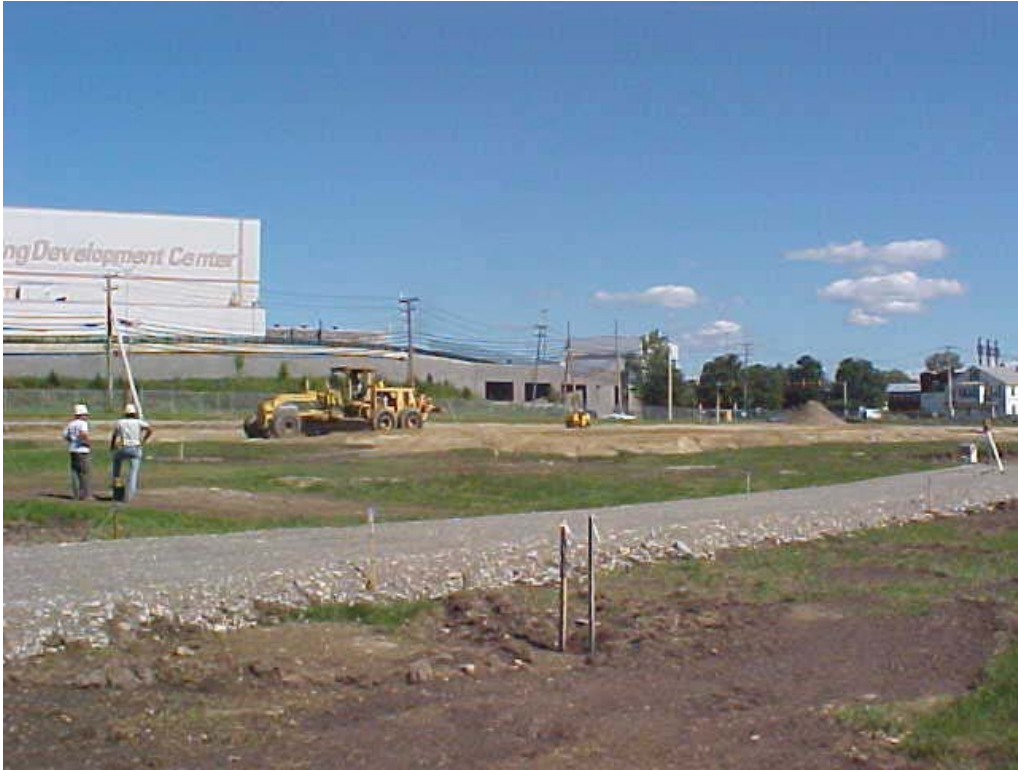
Photograph 17 Installation of the 1-foot-thick soil cover. The gravel subbase of the walking path is visible in the foreground. Photo taken looking northeast.
