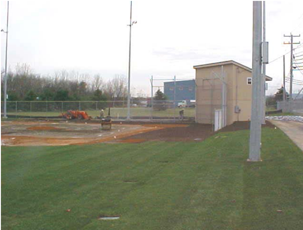
Photograph 21 Baseball field during placement of infield clay. Note the chainlink backstop. Photo taken looking west.
