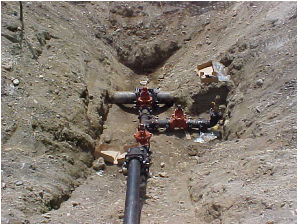
Photograph 4 Tie-in to existing water line. Note that the existing pipe downstream of the new tie-in (to the left of the tie-in in this photo) was later cut and capped due to leakage from the line.
