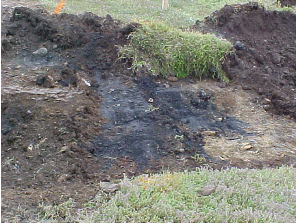
Photograph 13 Stained soil uncovered during excavation for light pole base at the northwest corner of the CRA just southwest of the scorer's booth.
