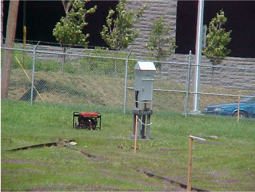
Photograph 3 One of the four air monitoring stations installed by Berkshire Environmental Consultants at the CRA. Photo taken looking north.
