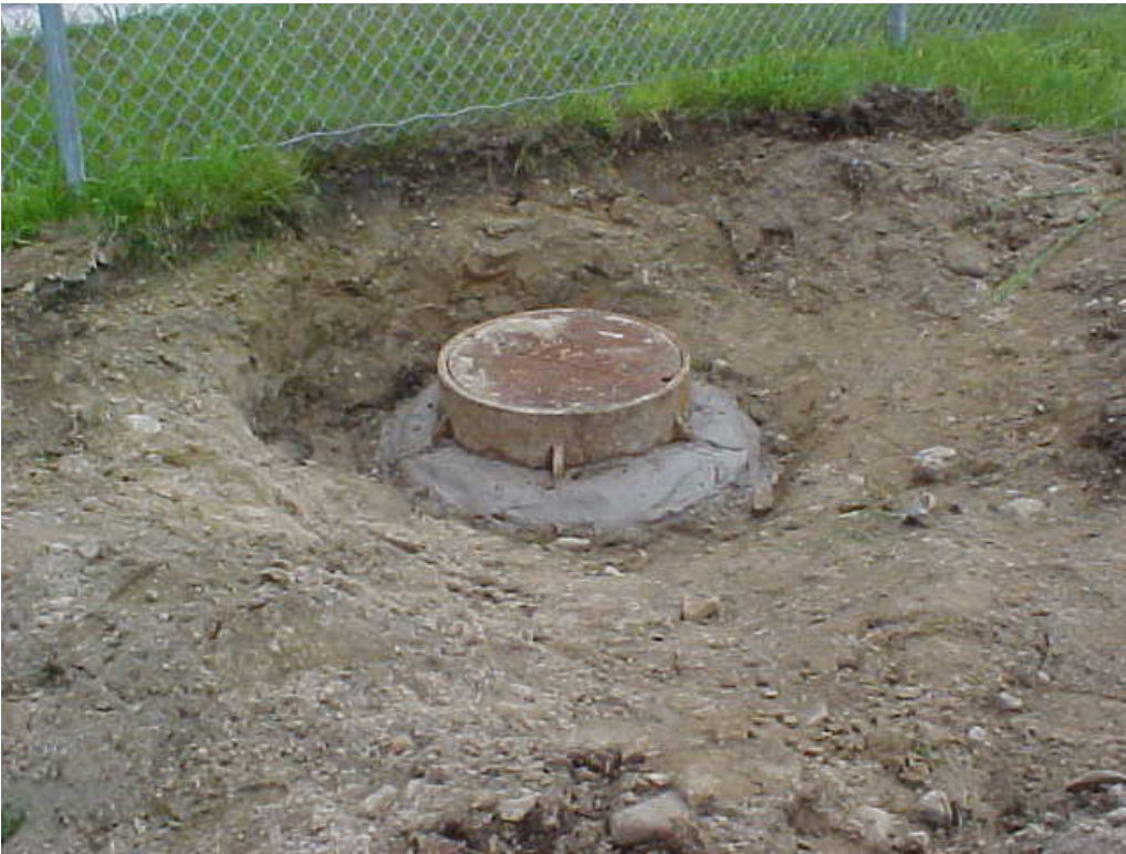
Photograph 14 Manhole ES-63 along the northern edge of the CRA. The frame and cover for this manhole were lowered approximately 1 foot and subsequently covered with geotextile and soil.
