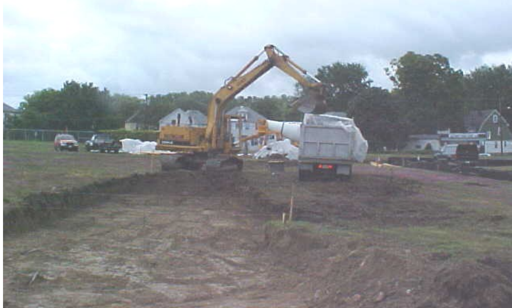
Photograph 7 Excavator loading a poly-lined dump truck with soil from the 2-foot removal area located at the southern edge of the CRA. Photo taken looking east.
