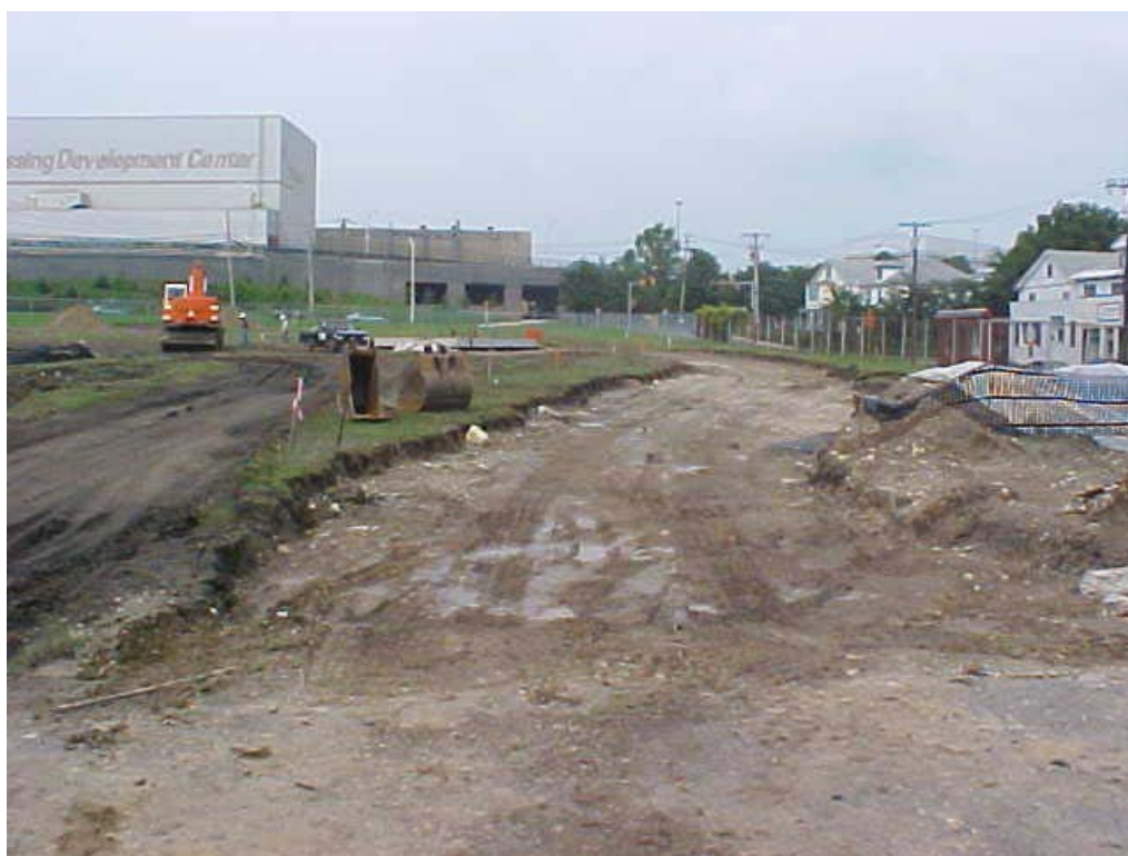
Photograph 10 Area of 1-foot soil removal for the access road. Photo taken looking north.
