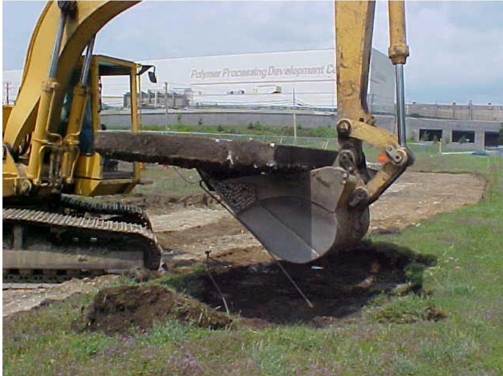
Photograph 8 Removal of a transformer pad located at the southeast corner of the CRA. Photo taken looking north.
