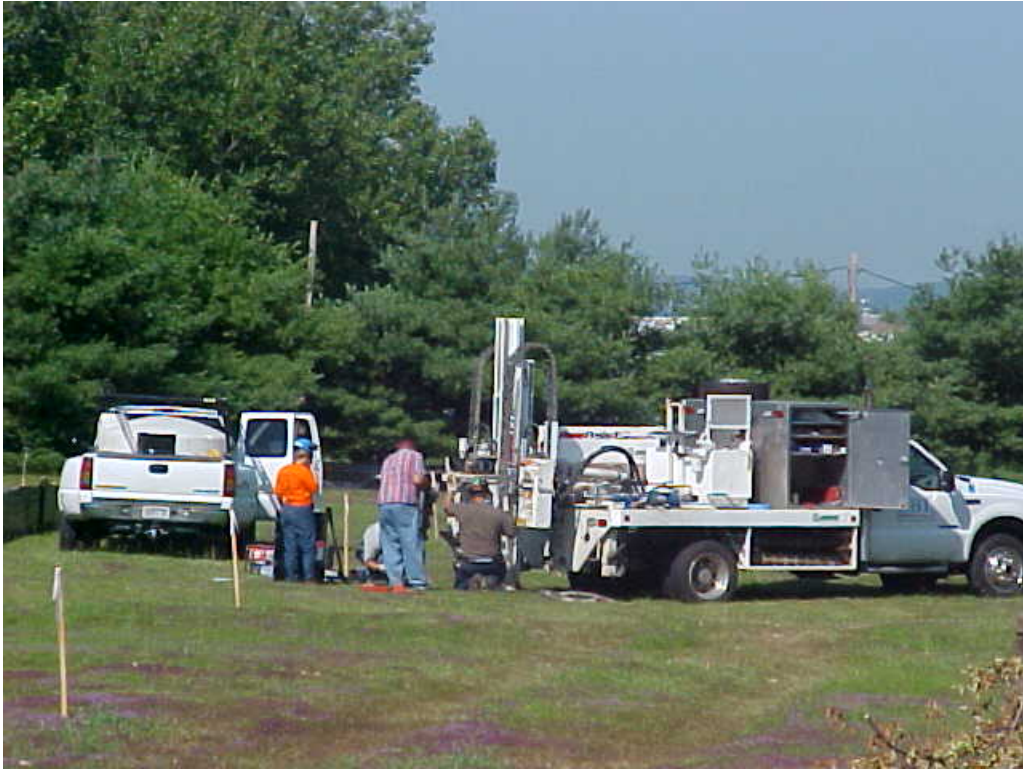
Photograph 5 BBL personnel with drill rig decommissioning monitoring well MW-66. Photo taken looking west.
