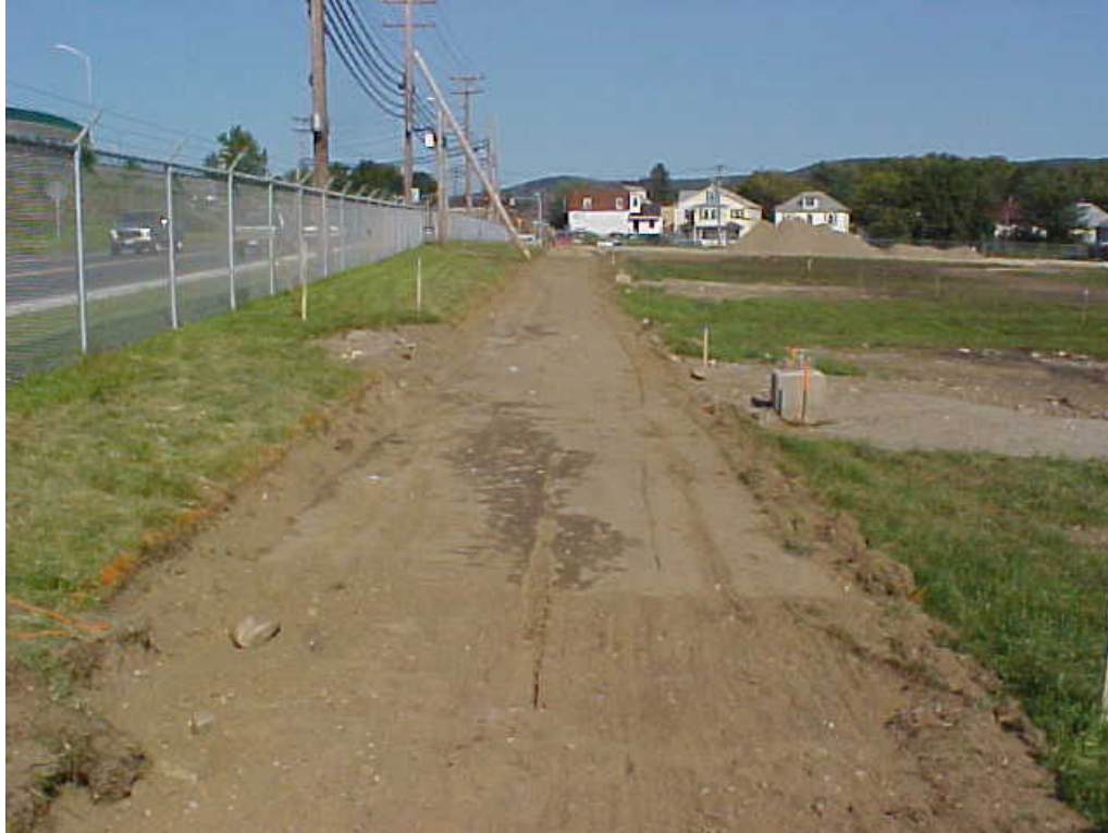
Photograph 16 The construction of the walking path along the northern boundary of the CRA. Photo taken looking east.
