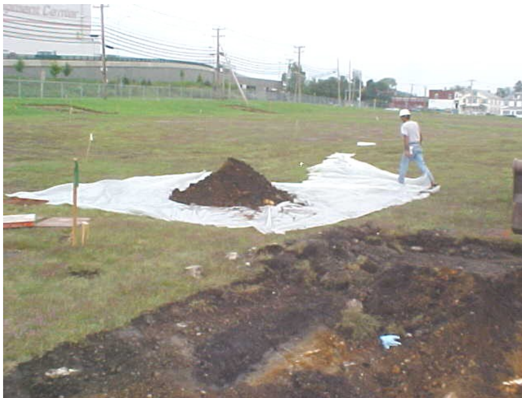
Photograph 9 Stained soil temporarily staged on poly. The soil was excavated from the area for the light pole foundation at the west side of the property, adjacent to first base. Photo taken looking east.
