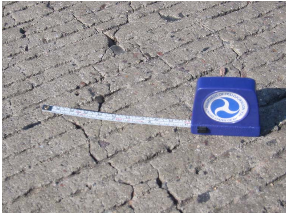
Figure 4. Example of pavement distress
