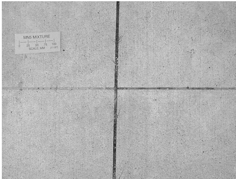
Figure 3. Photograph of Minnesota test section 5 (1998). Scaling is slightly heavier than figure 2, and in some areas the surface texture (brooming) is obscured.
