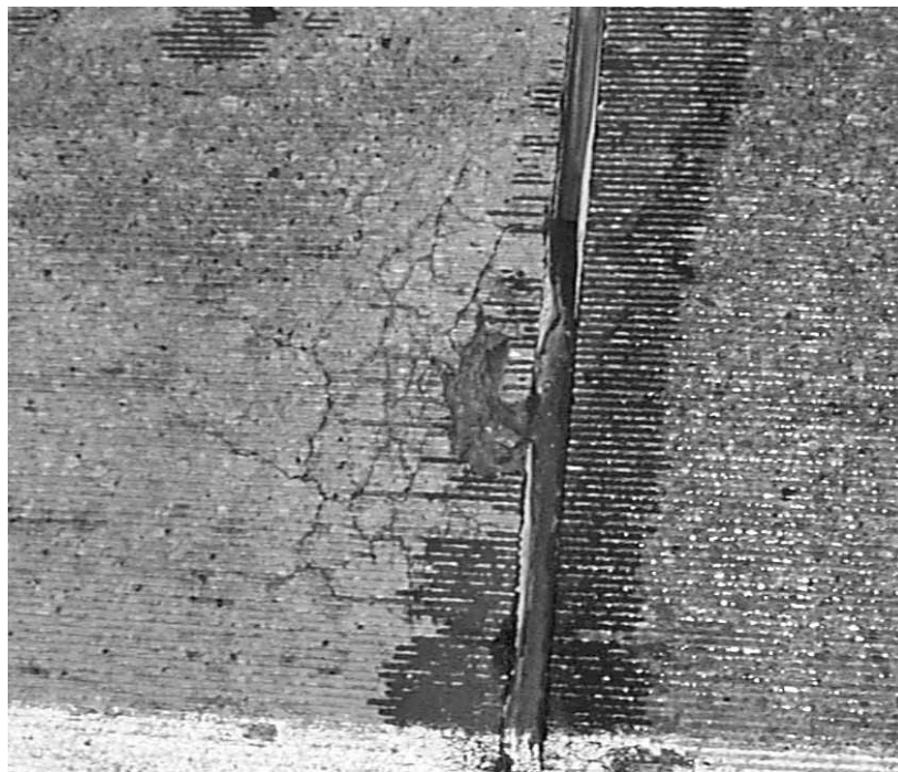
Figure 5. Deterioration in patch (left) in wheelpath, mixture I4 (surface has been diamond ground, and note longitudinal paint strip along pavement edge at bottom of photo).
