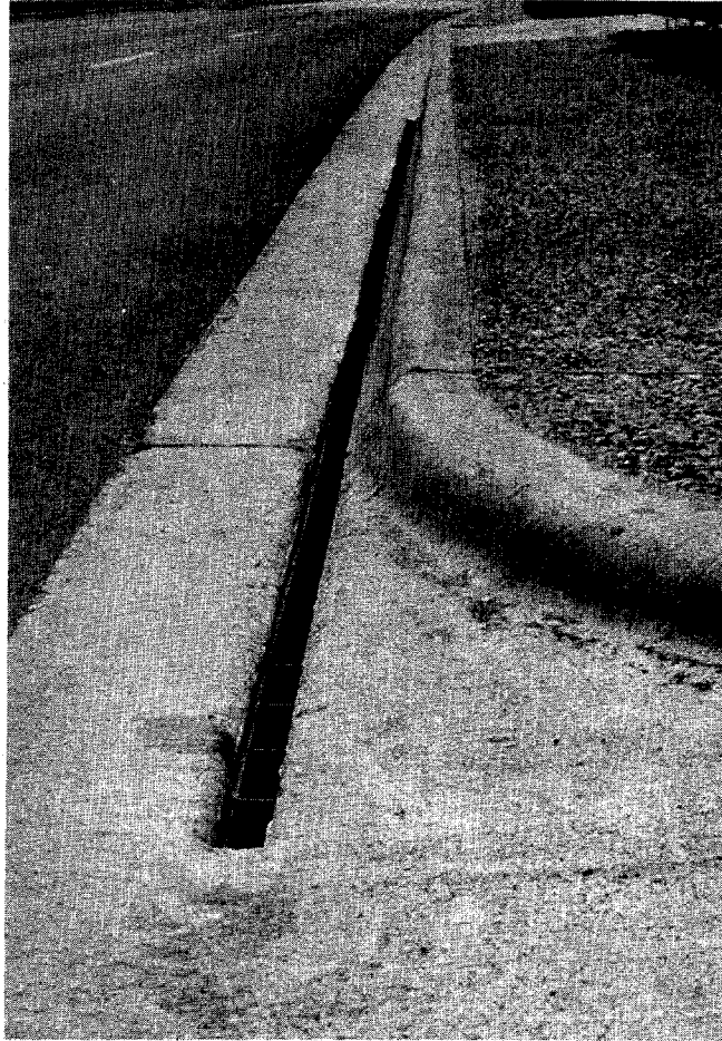
Figure 18. Slotted drain inlet at an intersection.
