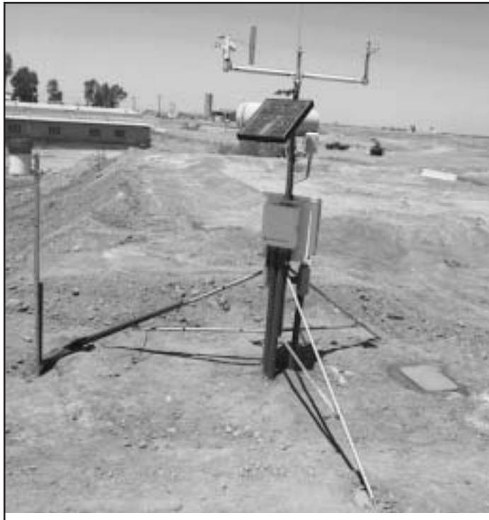
Installed weather station & datalogger.
