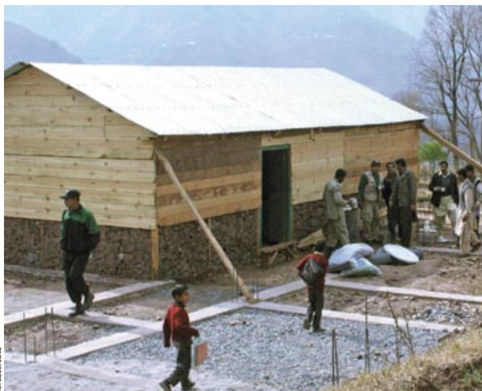
NEW HOUSE —Villagers in Langla along the Jhelum River in Pakistan-controlled Kashmir stand near a new home built on the foundations of a house destroyed in the earthquake. USAID supplied the metal roofing sheets, other materials, tools, and know-how. It is earthquake-resistant, its wooden structure made from heavy beams that were sawn into thinner boards.
