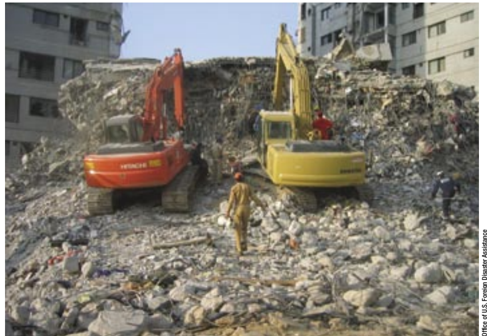
Parts of the Margala Towers condominium complex in Islamabad sustained significant damage during the Oct. 8 earthquake that struck the South Asia region. USAID's Disaster Assistance Response Team conducted an assessment of the buildings as part of its work in Pakistan.
