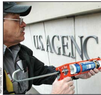
Workman attaches sign for USAID on the 14th Street face of the Ronald Reagan Building Dec. 9 in Washington, D.C., seven years after the move from the State Department into the new building.
