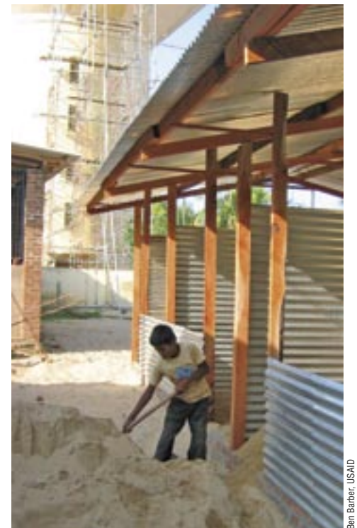
A boy works on a temporary housing project for Sri Lankans displaced by the tsunami.
