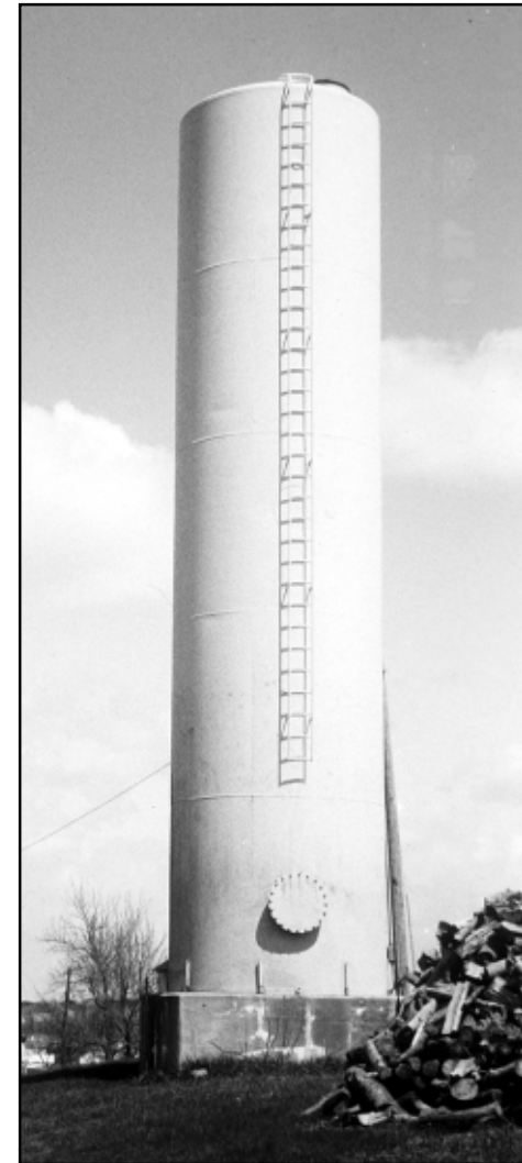
Standpipes such as this one are an example of the types of projects to benefit small drinking water systems that are eligible for CoBank funding.
