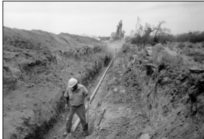
Among the uses of HUD Community Development Block Grants is funding the replacement of pipes that distribute drinking water to the customers of small rural systems.
