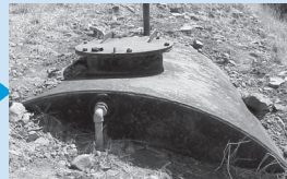
Storage and Distribution
