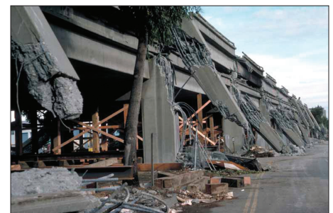
The upper level of this two-level section of Interstate 880 in Oakland, Calif., collapsed during the magnitude 6.9 Loma Prieta, Calif., earthquake on October 17, 1989. Forty-one motorists were killed in the collapse (USGS photograph).
