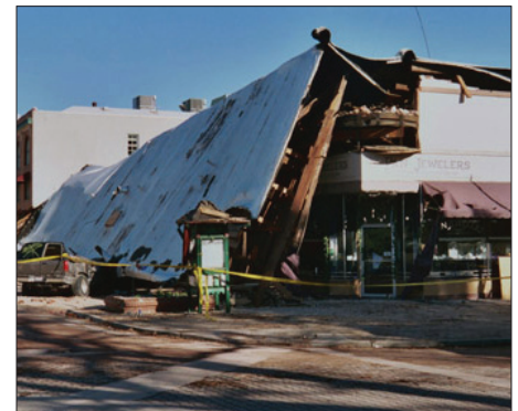
A vehicle, seen near the left edge of this image, was crushed under this collapsed storefront in Paso Robles, Calif., during the magnitude 6.5 San Simeon, Calif., earthquake on December 22, 2003. Two people were killed trying to get out of the store during the earthquake (FEMA photograph/Dane Golden).
