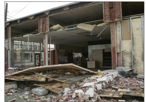
This business in Seattle was heavily damaged during the magnitude 6.8 Nisqually, Wash., earthquake on February 28, 2001. About 400 people were injured during the earthquake (FEMA photograph/Kevin Galvin).
