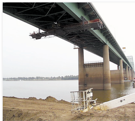
Figure 6. Effective strengthening of existing structures, like the recent retrofitting of the I-40 bridge crossing the Mississippi River, requires accurate information about likely earthquake ground shaking. (Photo by G. Patterson, CERl, University of Memphis.)
