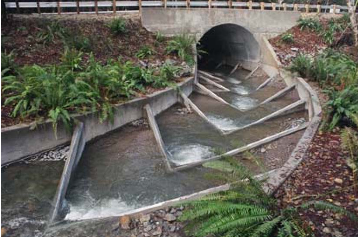
Figure 7.17 Fishway installed on Peacock Creek, California (Llanos 2004)
