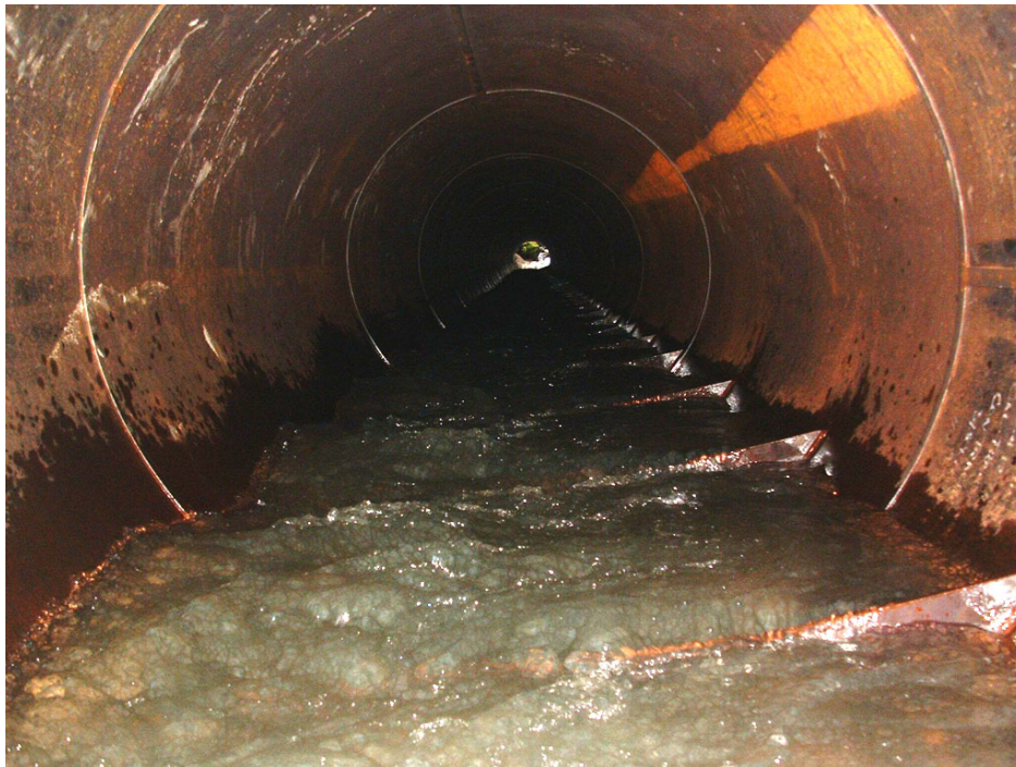
Figure 8.15 Baffles slowing water velocities at high flows while producing minimal turbulence, John Hatt Creek
