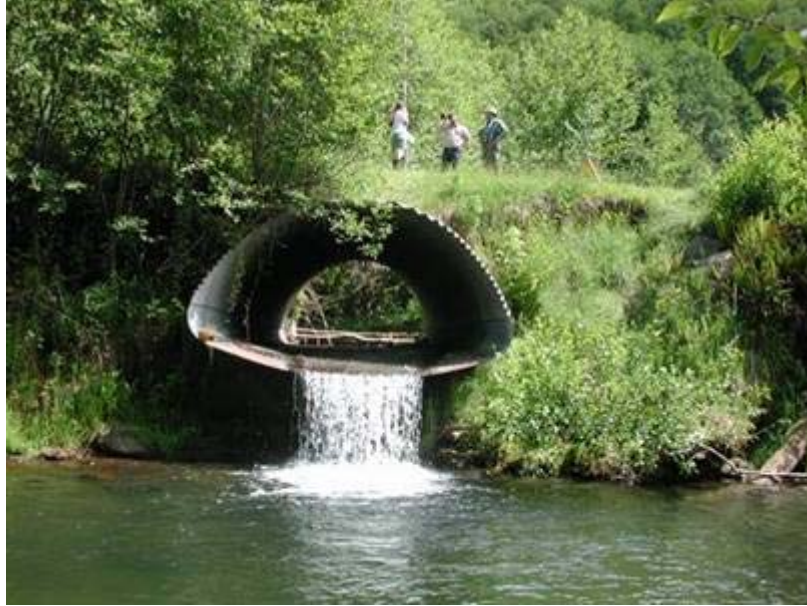
Figure 1.2 Downstream channel degradation causing culvert to become perched, and presenting a low flow barrier to fish passage (Furniss 2006)
