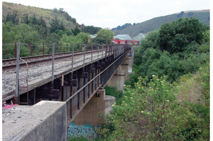
Figure 2-20. The original railroad bridge over the Pajaro River was heavily damaged by the 1906 earthquake. The bridge straddles a strand of the San Andreas Fault, which caused minor rotational offset of the bridge during the 1906 earthquake. The area also experienced heavy shaking during the 1989 Loma Prieta earthquake. Piles of gravel from the Logan Quarry are in the distance.
