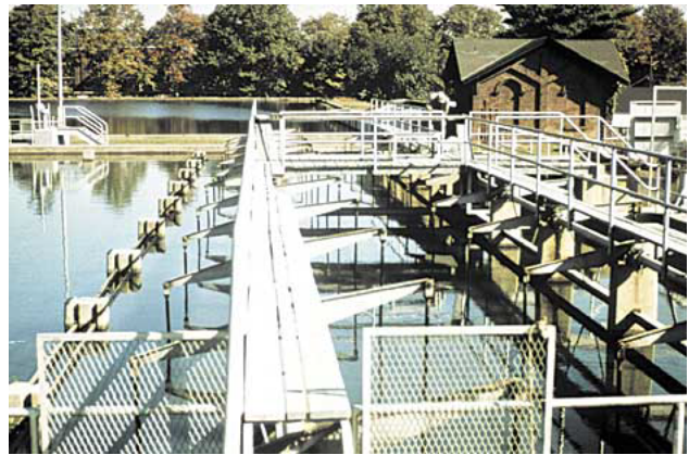
Wastewater treatment plant, New Brunswick, New Jersey (Photograph by Eric Vowinkel)
