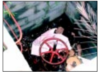
Valve on Chamelco River. La Lima, Honduras
