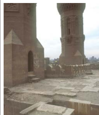
The upper terraces of the gate and the bases of the minarets, before and after restoration.
