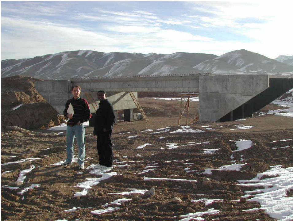
A photograph of RIG/Manila auditors viewing one of six bridges under construction on the Kabul to Kandahar highway. A paved detour allows traffic to circumvent the construction area until the bridge is complete. This photograph was taken in January 2004 about 48 kilometers outside Kabul, Afghanistan.
