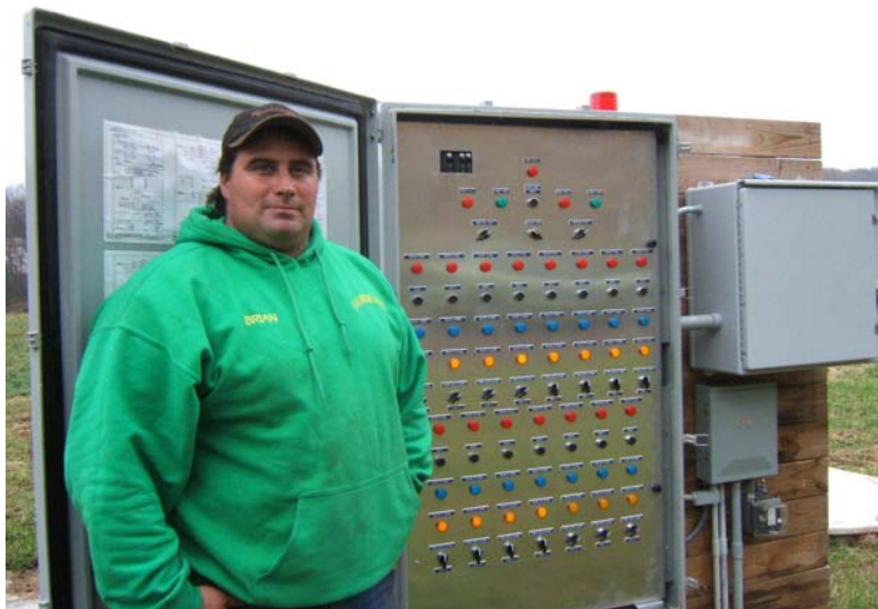
Figure 1.13 Brian McIntosh, operator of the new Bovina Community Septic System, at the control panel, where flow from the settling tanks is directed to twelve leach fields. Photo courtesy of Catskill Watershed Corporation
