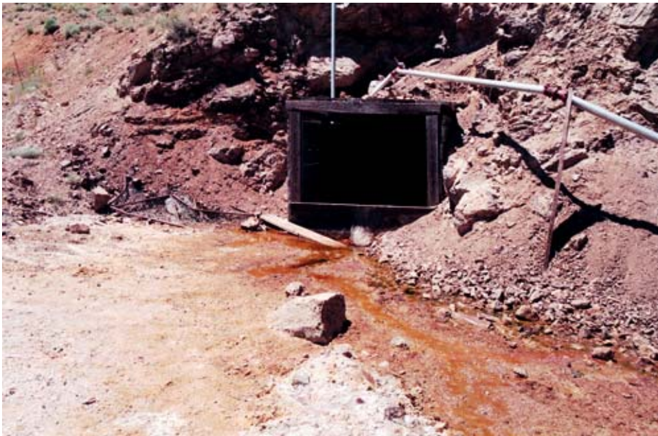
Photograph 6. Drainage from this mine tunnel reacts with sulfidic waste to create even more acidic (pH 2.6) water and extremely high metal concentrations. The adit was plugged and the dump was reclaimed in 1998.
