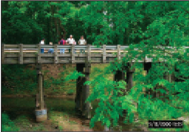
Bridges that span entire riparian areas at floodprone width instead of just the active stream channel width allow larger wildlife species such as deer and bear to pass safely under roads.
