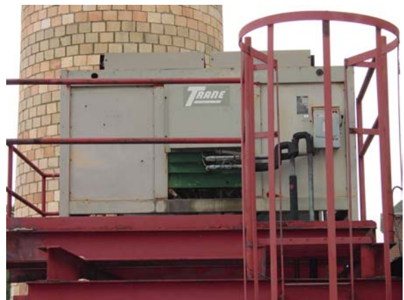
Figure 38. Air-handler unit for first floor located on boiler house.
