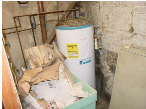
Figure 27. Hot water tank/storage room.
