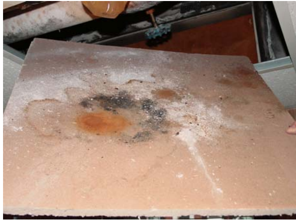
Figure 14. Back of ceiling tile from District Attorney's basement office.
