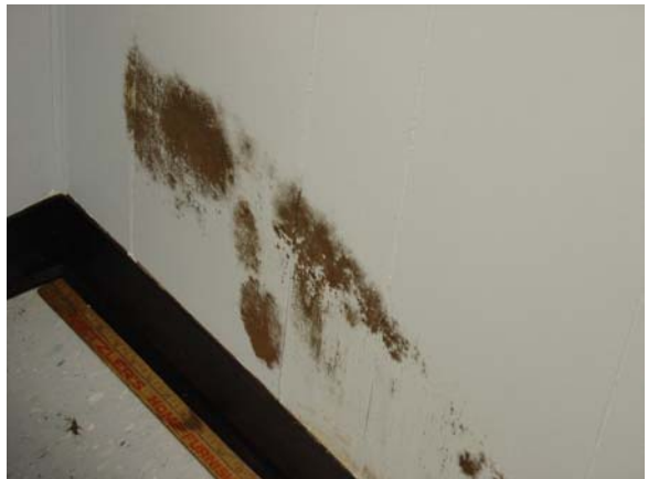
Figure 16. Potential mold on wall in Coroner's office.
