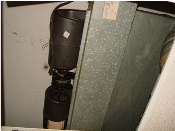
Figure 35. Snack room fan-coil unit.
