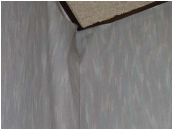
Figure 19. Wallpaper coming away from wall behind the door in the Clerk of Courts’ office.
