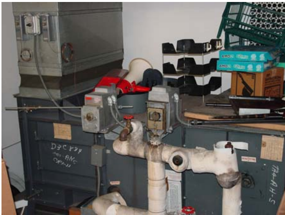
Figure 39. Air-handler unit for Sheriff's office located in confiscated weapons lock-up room.
