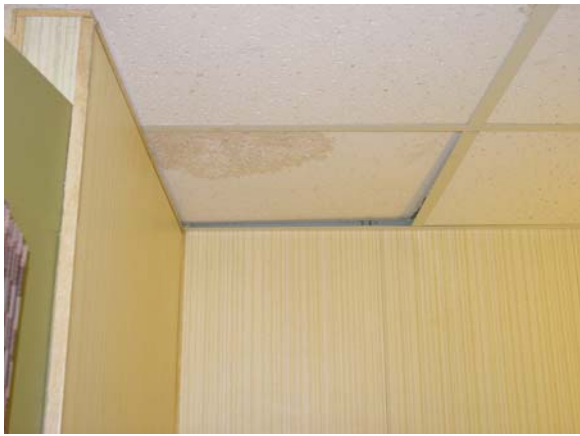
Figure 11. Ceiling tile in Treasurer's office.
