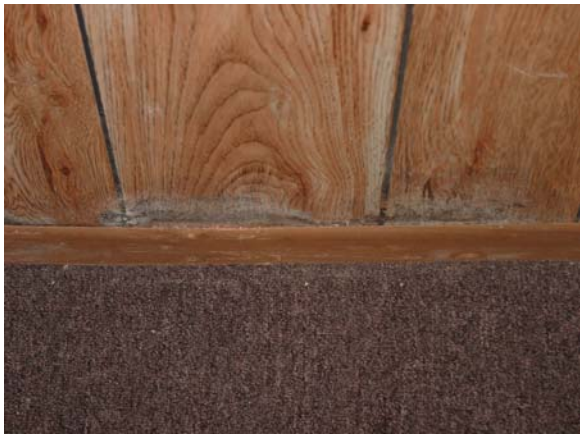
Figure 17. Possible mold on paneling in Assistant District Attorney’s office.
