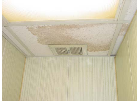
Figure 10. Ceiling tile in Controller's office.
