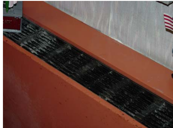
Figure 20. Vent in Clerk of Courts’ office with white powder from beneath the wallpaper.
