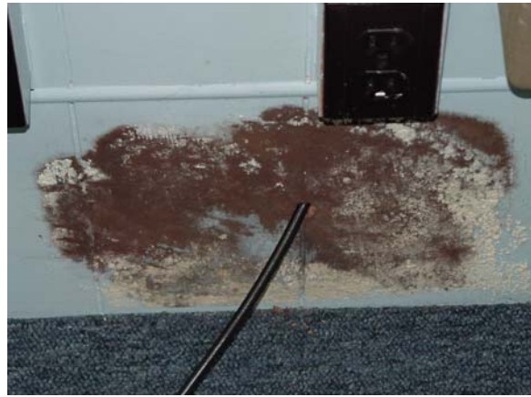
Figure 30. Boroscope being used to investigate the inside of the arch wall in the Coroner's office.
