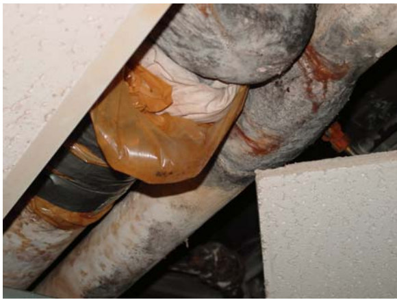
Figure 37. Plastic wrapped around leaking pipe in District Attorney's basement office.
