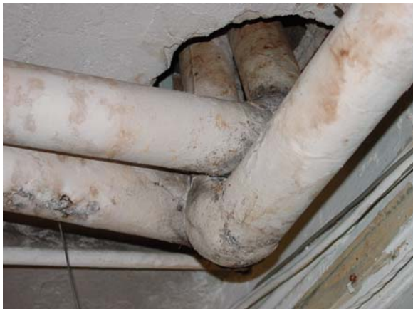
Figure 15. Overhead steam pipes in Clerk of Courts' basement storage room.
