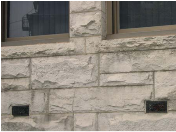
Figure 23. Possible openings under Clerk of Courts' office windows.
