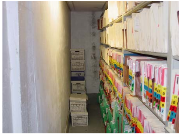
Figure 18. Inside of exterior wall in Clerk of Courts’ basement storage area.
