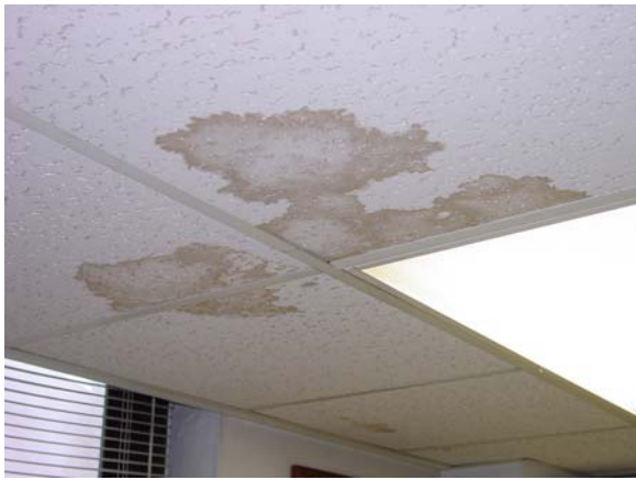
Figure 7. Ceiling tile in Public Defender's office.
