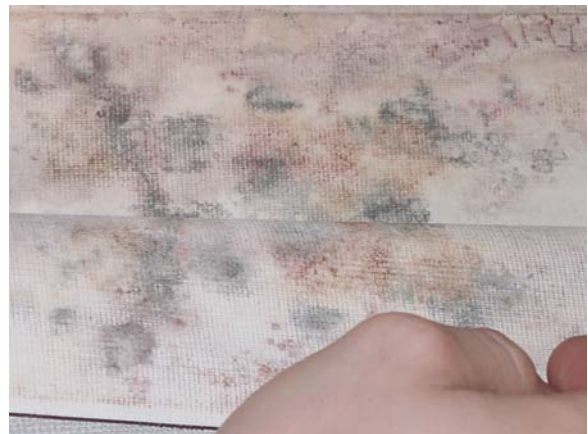
Figure 22. Possible mold on back of wallpaper in Clerk of Courts’ office.
