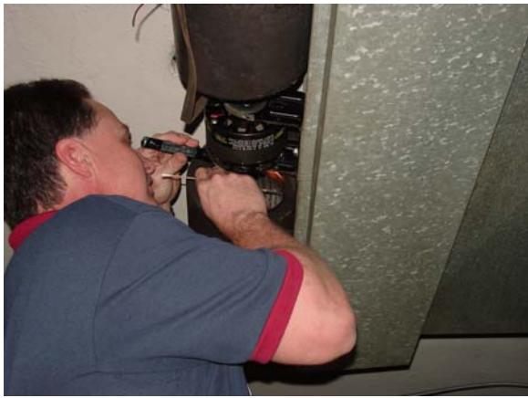
Figure 5. Swab sample being taken from fan-coil in ceiling of snack room.
