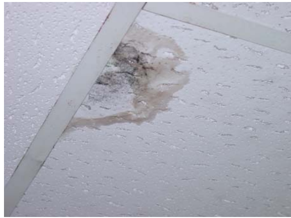
Figure 6. Ceiling tile in Lower Commissioner's office.
