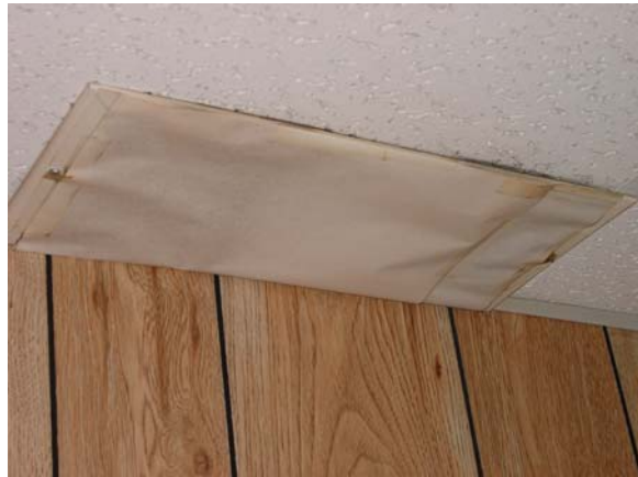
Figure 26. Covered vent in Witness room.
