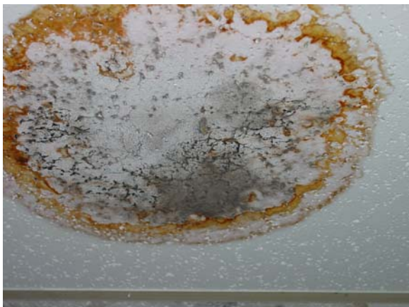
Figure 9. Ceiling tile in Witness Waiting Room.
