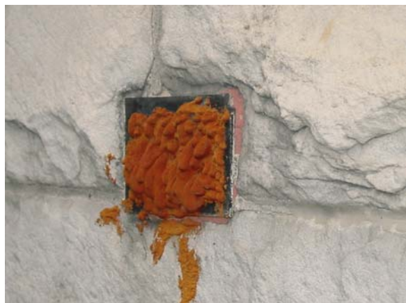
Figure 24. Plugged opening under Clerk of Courts' office window.
