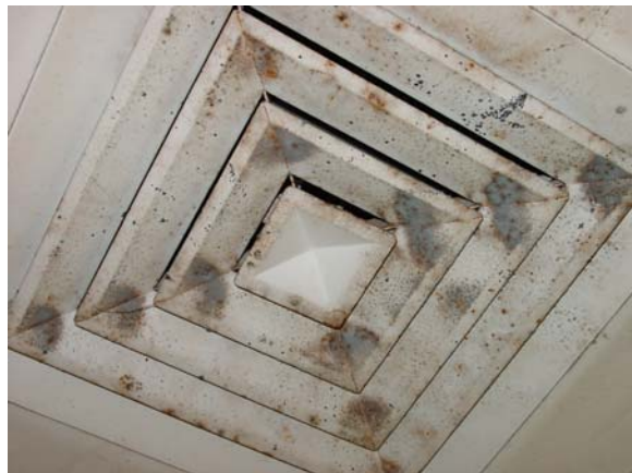
Figure 13. Vent in Witness room.
