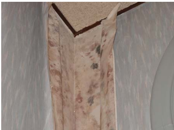
Figure 21. View of wall behind bulging wallpaper in Clerk of Courts’ office.
