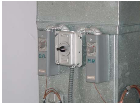
Figure 40. Outside/return air controller.
