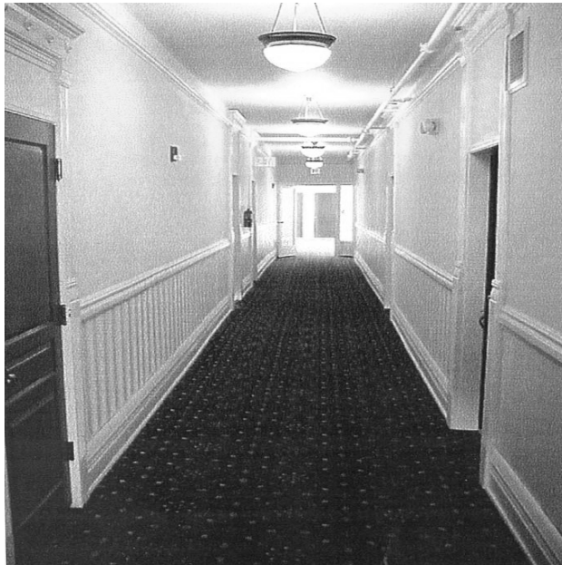
Bostwick 6.16: The corridors of the Bostwick Building were rehabilitated to their historic appearance.
