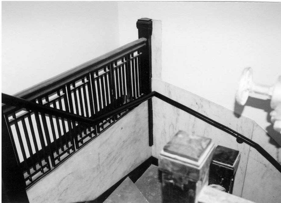
Chambers 6.12: One of the few historic interior features remaining in the building, the historic steel stair was repaired and retained. Windows openings adjacent to the stair, located on a secondary elevation, were enclosed in order to allow the stair to be used as a fire exit.
