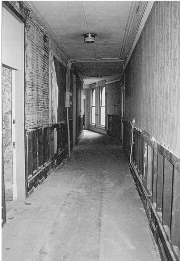
Bostwick 6.15: As seen in this photograph of a corridor, previous owners removed much of the building's decorative woodwork. Fortunately, the material was stored on-site and was reinstalled during the rehabilitation.
