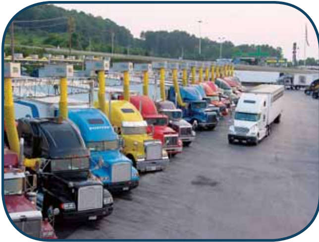
The Petro Travel Center in Knoxville, TN provides advanced truck stop electrification, limiting emissions.
