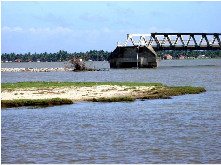
The bridge over Arugam Bay was destroyed by the tsunami. Its replacement is the largest of three USAID projects under a contract signed September 7. Photo: USAID/Lionel Jayaratne
