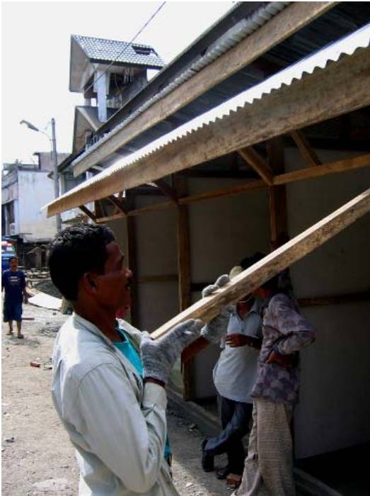
Banda Aceh Market Rehabilitation laborer at work. Photo: Paul Dillon from International Organization of Migration/Banda Aceh
