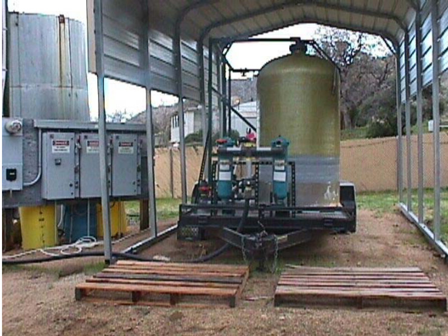
Figure 4-5. Trailer-Mounted HIX System under a Canopy
