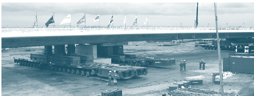
Figure 14(a). SPMTs lift two-span bridge crossing Amsterdam’s A4/A5 expressway off temporary supports. COURTESY OF MAMMOET
