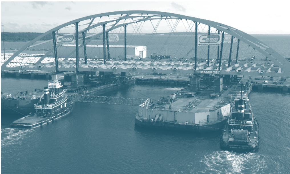
Figure 11. SPMTs move RIDOT Providence River bridge span onto barges at staging area.
