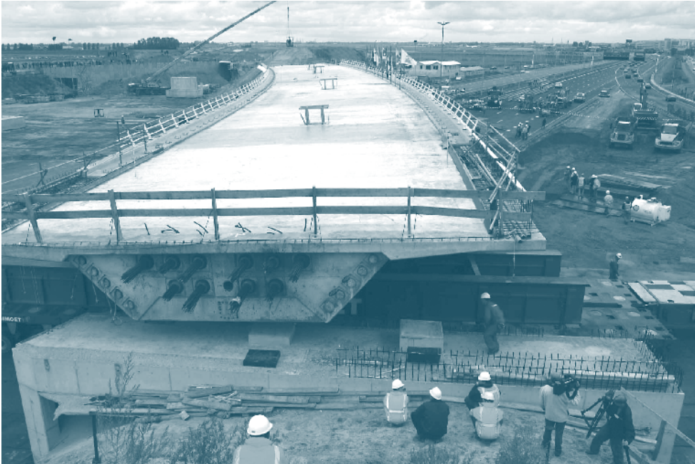
Figure 14(b). SPMTs move bridge crossing Amsterdam’s A4/A5 expressway to final location. COURTESY OF MAMMOET
