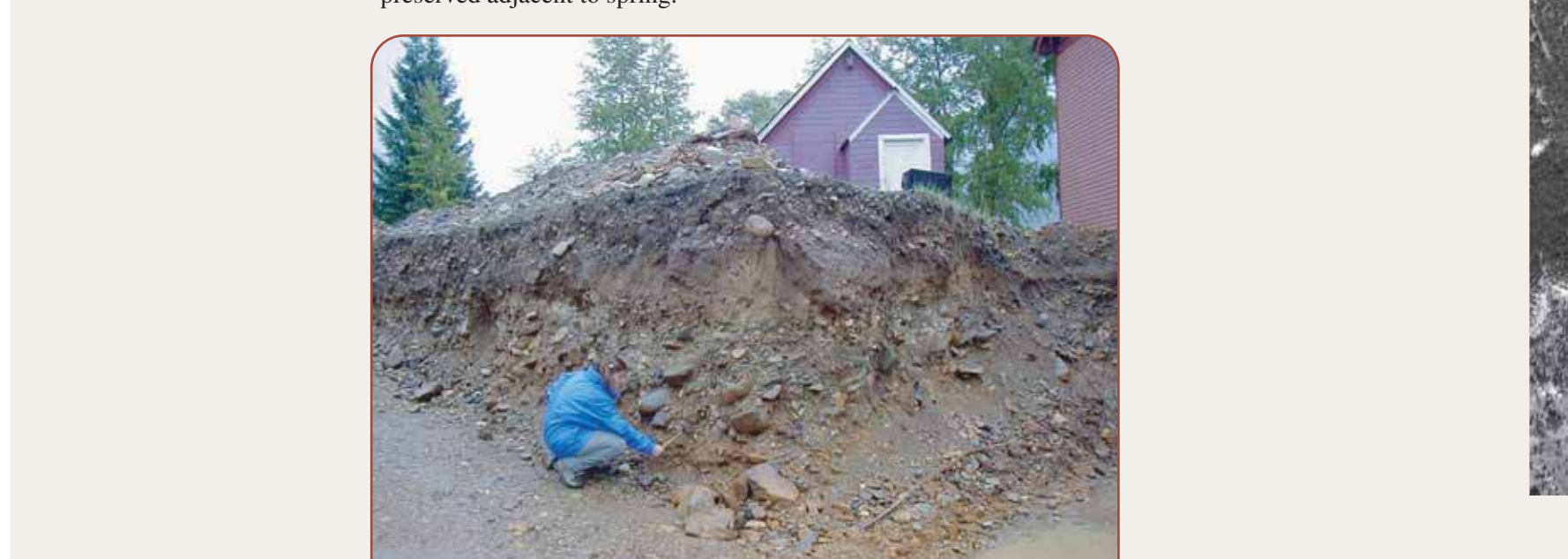
Figure 8. Alluvial ferrite east of excavated foundation (town of Silverton). Builders commonly encounter ferrite 'hardpan' when excavating foundations throughout the town.
