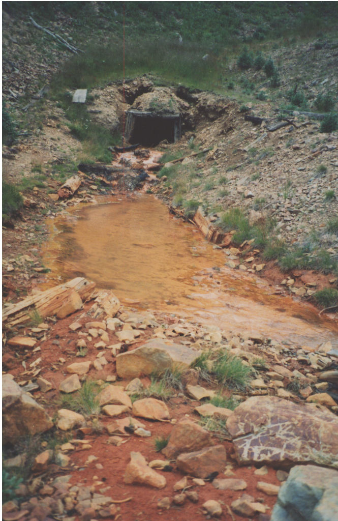
Figure 14. Collapsed adit of Natalie/Occidental mine releases one of the larger flows of mine water in the study area. Metal concentrations of the pH 6 water are not unusually high, but because of the high flow rate, loads of copper and zinc are high. Adit is about 1½ m across.
