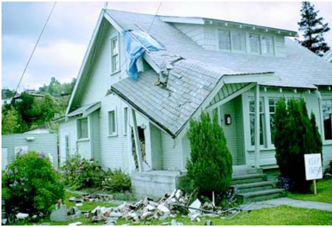
FIGURE 3. Chimney damage to single-family house as a result of the 1965 Seattle-Tacoma Puget Sound earthquake (Reprinted with permission from the Karl V. Steinbrugge Collection, Earthquake Engineering Research Center ).
