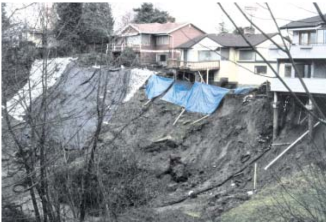
FIGURE 1. Landslide in northwest Seattle. Foundation of house on right edge of photograph and decks of neighboring houses have been undermined. (Photo by Alan F. Chleborad, USGS , January 9, 1997.)
