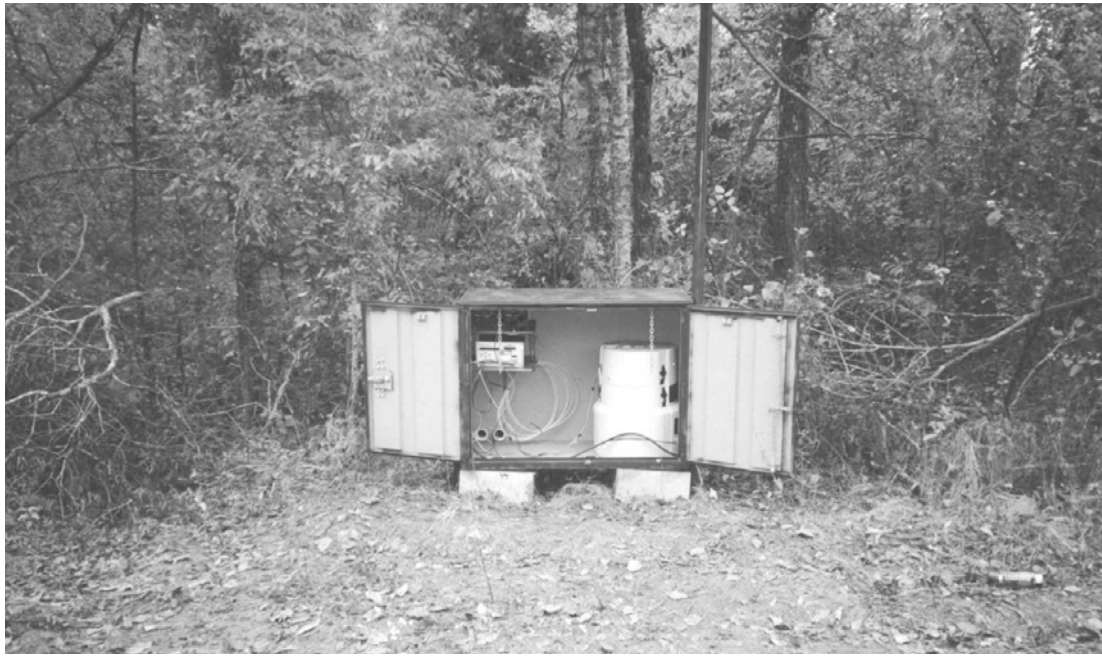
Figure 3. Forested storm monitoring station at Boeuf River Diversion Canal near Hudspeth, Arkansas.
