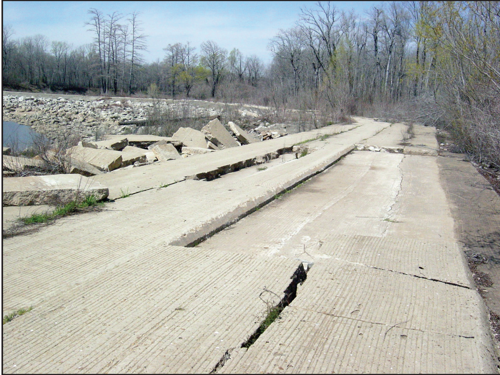
Figure 9. Melinda Head Cut Structure looking toward the northwest. Concrete slabs located toward the water were transported by flood water from the White River. Photograph by John B. Czarnecki, U.S. Geological Survey.
