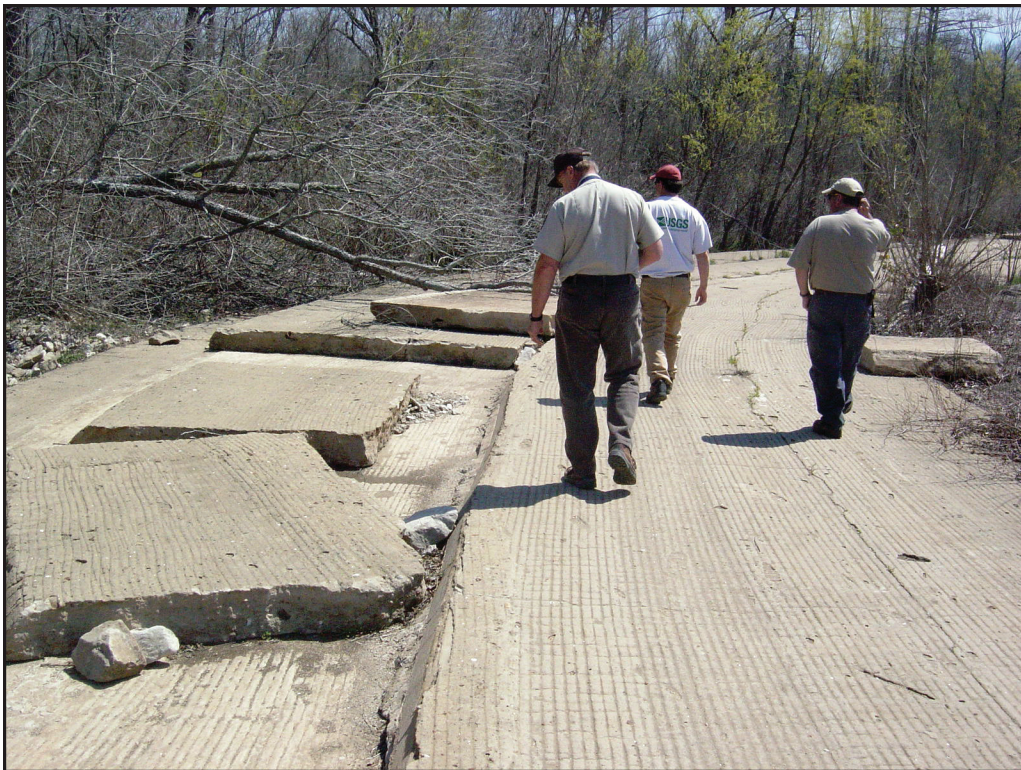
Figure 10. Damage along the top of the Melinda Head Cut Structure, spring 2005. Concrete slabs were removed by the force of flood waters from the White River, which covered the Melinda Head Cut Structure. Photograph by John B. Czarnecki, U.S. Geological Survey.
