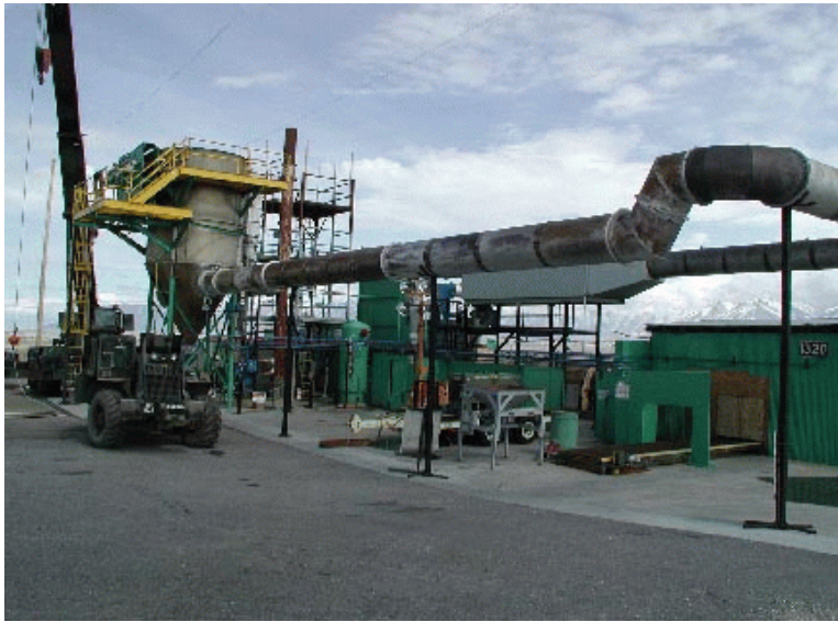
Figure 3-1. Deactivation Incinerator at TEAD
