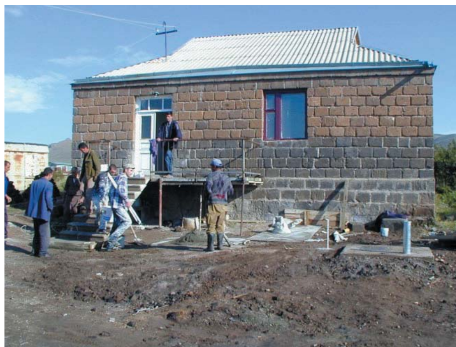
Construction workers finish the last details as an Armenian family prepares to move into its newly constructed home in its own village with the help of USAID-sponsored housing program.
