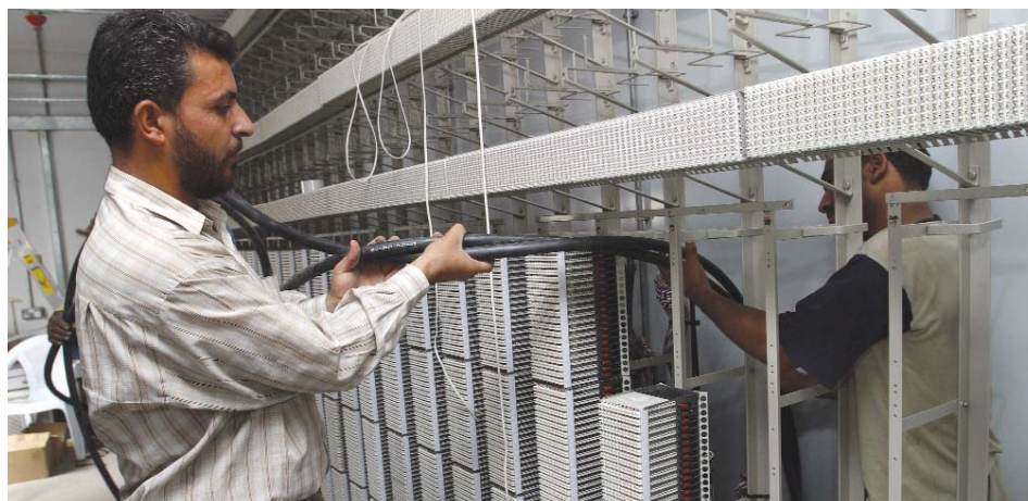
Thomas Hartwell, USAID Repair work at the Al-Mamoun telephone exchange, Baghdad. Bechtel has been working with the Iraqi Telephone and Postal Company to restore telephone service.
