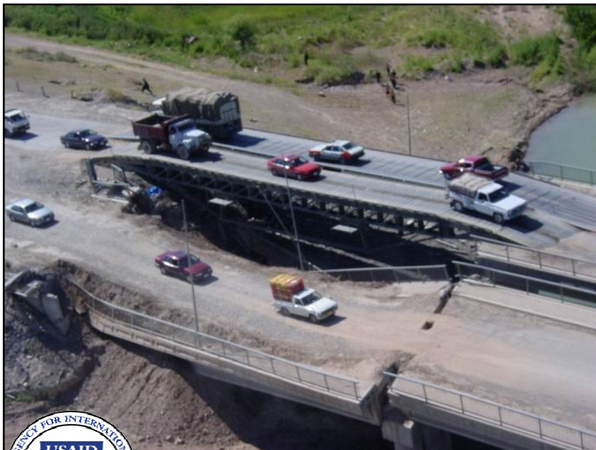
The reconstruction of the Khazir Bridge, a four-lane bridge in northern Iraq, was complete in early April.
