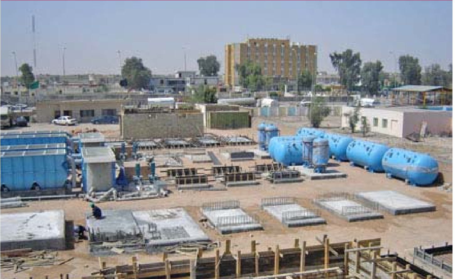
When complete in September, the Karbala water treatment plant will serve millions of residents and religious pilgrims.
