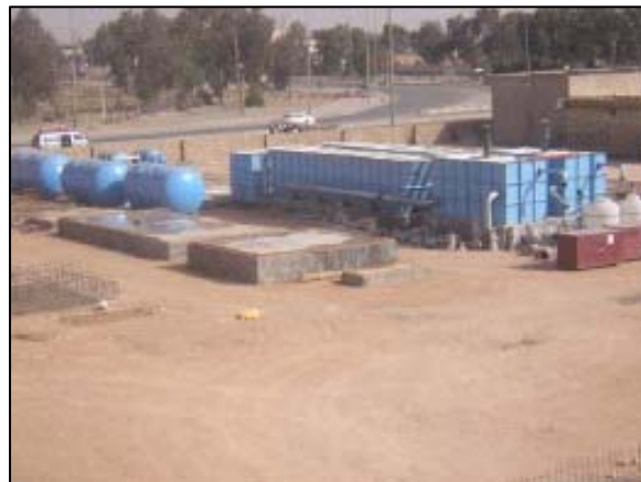
Workers are continuing to build foundation pads for compact water treatment units.
