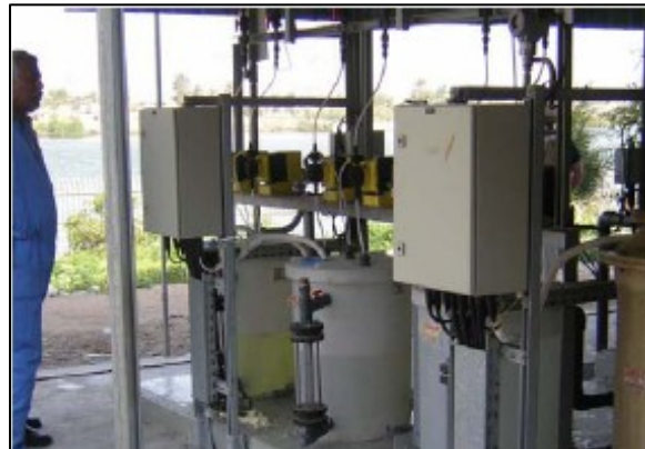
Newly installed desalination equipment will improve the plant's efficiency.
