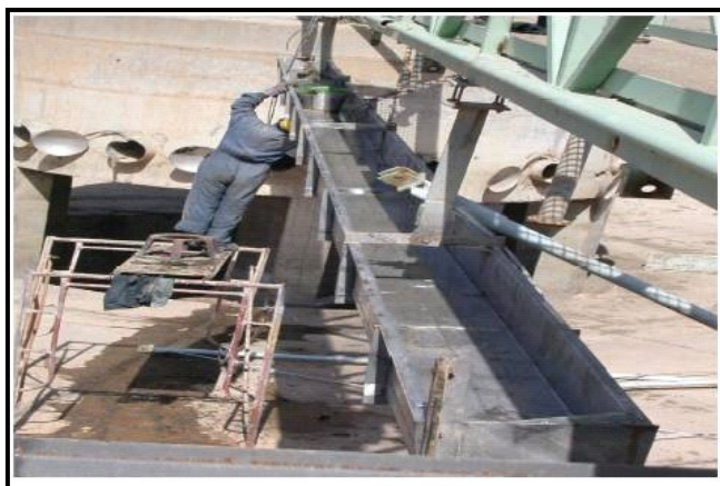
Repairing skimmer in primary settling tank at Rustimiyah North, one of three wastewater treatment plants in Baghdad.
