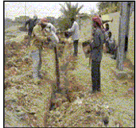
Workers at Al-Mullah Ahmad village preparing to lay a water distribution pipe.
