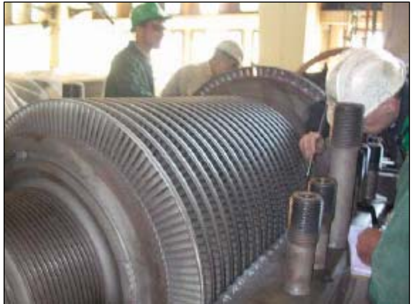
Work is now 81% complete on the refurbishment of two units at a Baghdad power station.
