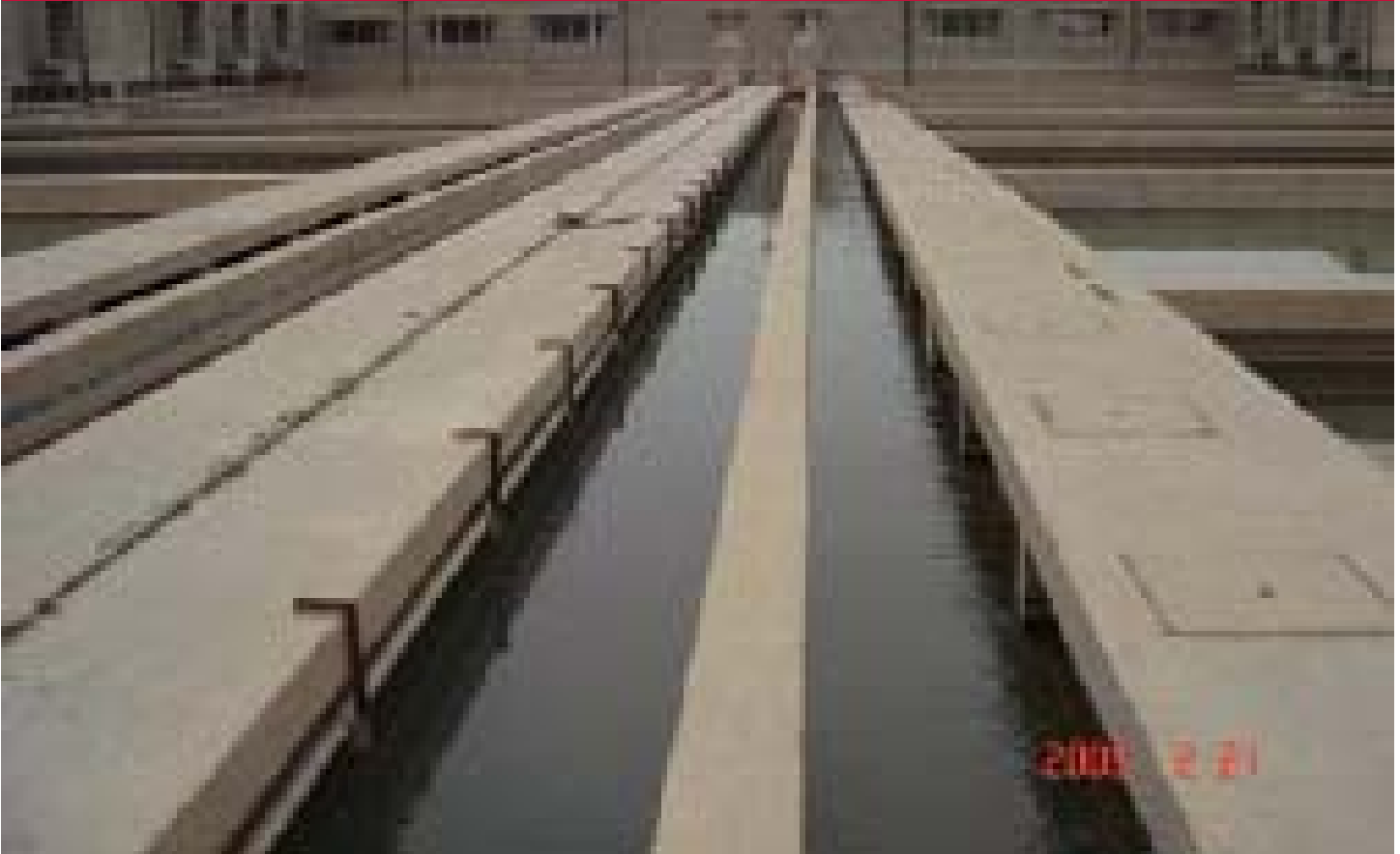
The expansion and rehabilitation of the Sharkh Dijlah water treatment plant is helping to address a water shortage in Baghdad.
