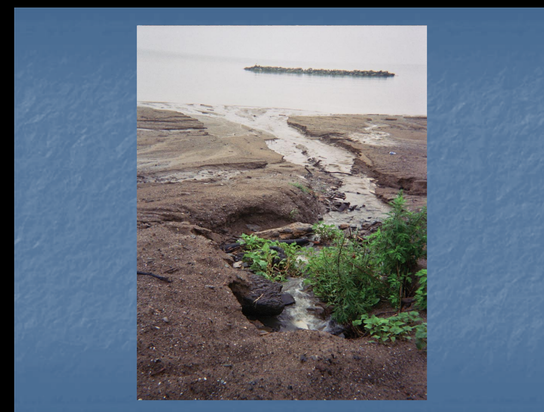
Figure 3. On July 12, 2004, it rained 0.68 inch between 6 and 8 a.m. The field crew observed the formation of a conduit to the beach from a pipe draining the parking lot. The E. coli concentration from the flowing pipe was 26,000 col/100 mL.
