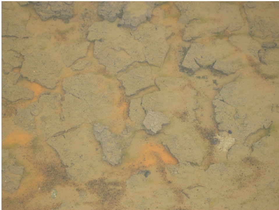
Figure 22. Carbonate and iron-rich ground water seepage. Note also faint regions of green material and the nonuniformity of iron (orange) and green coloration, December 2006.
