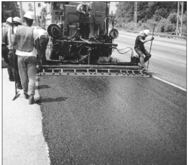
Georgia DOT has recently added microsurfacing to its arsenal of preventive maintenance treatments.
