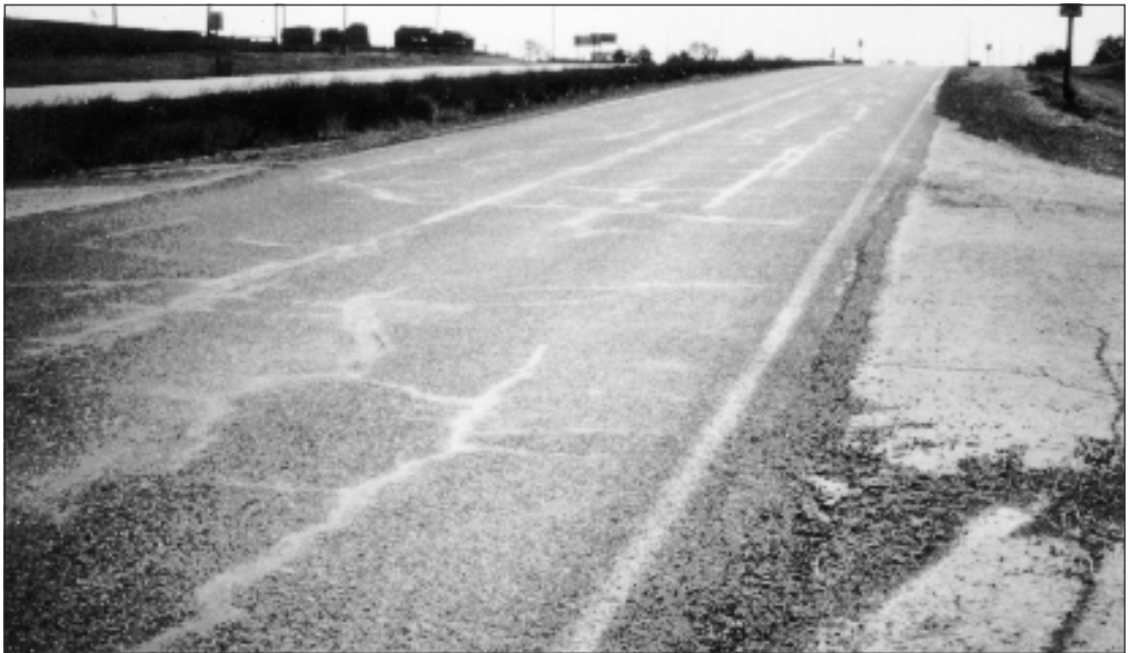
Kansas DOT applied chip seals and crack seals to Route 68 in Ottawa, producing one of the State's best-performing pavements. The treatments were not only effective, but also very inexpensive.
