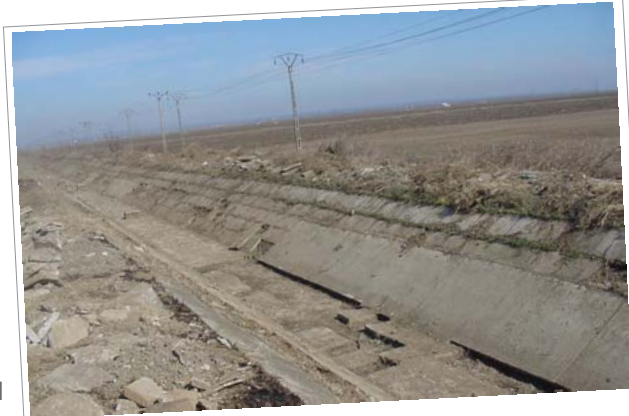
Irrigation ditch in need of repair
