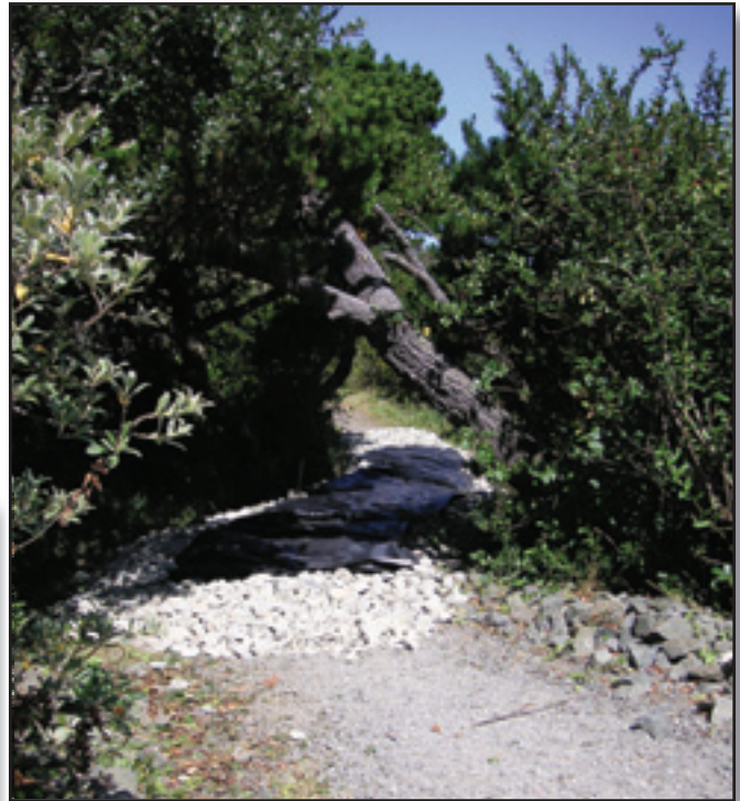
Figure 21—Constructing an underdrain from large rocks, with geotextile serving as a separator between surface material and large rocks.
