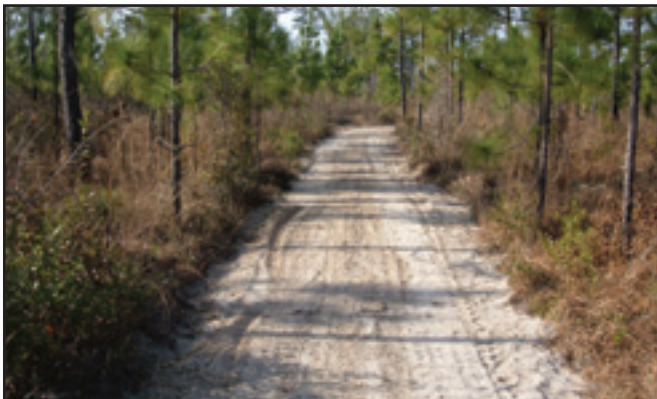
Figure 17—The finished trail after Geoblocks were installed in the Francis Marion National Forest.
