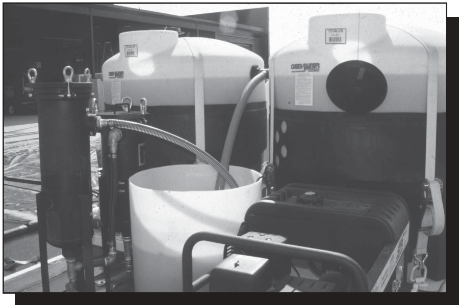
Figure 6—Two cone-bottom tanks are used as settling tanks to remove the larger particulate. The overflow from each tank is pumped through two filters and then to the holding tank.
